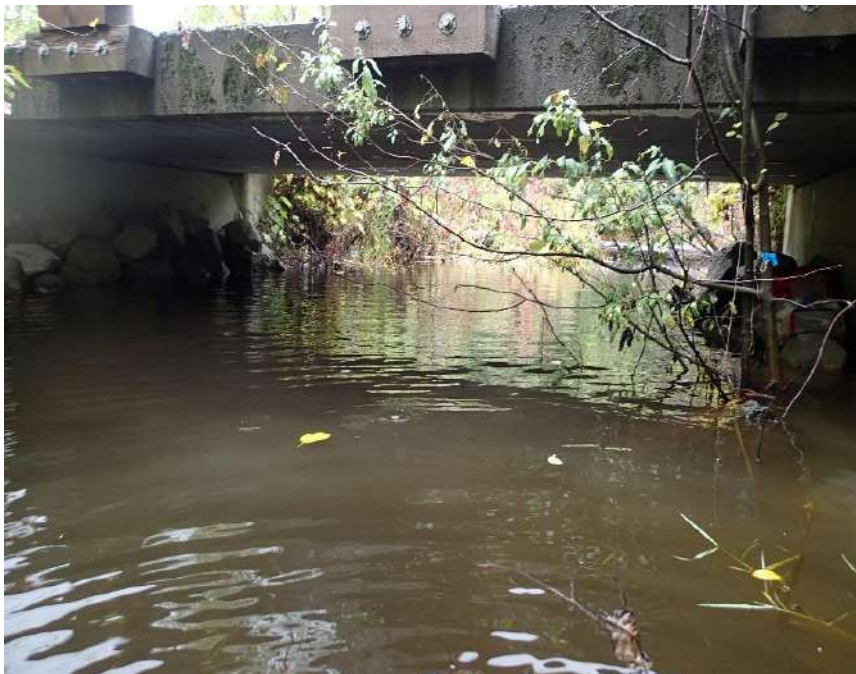
Figure 6. Looking upstream at ALE-BDGWQ on September 27, 2021.
