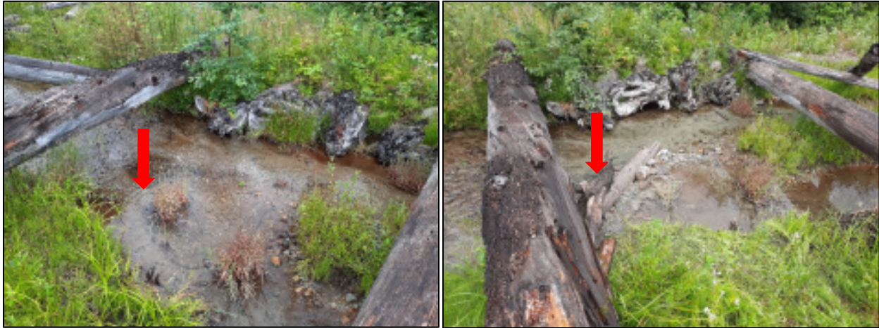
Figure 11. Instream repair near ALE-XS6, before (left) and after (right) repair. Flow is from right to left. Rock/wood flood deflector was installed to scour sand deposited under root wads and to focus flow back into the original channel alignment.
