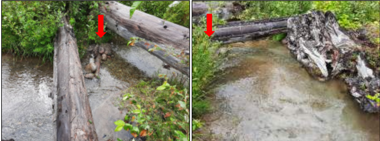
Figure 13. Flow deflector and bank stabilization installed at ALE-XS6, after repair. Flow in left photo is from right to left and arrow shows new deflector. Flow in right photo is from left to right and shows how redirected flow energy has already begun to clean out material deposited at base of root wads.
