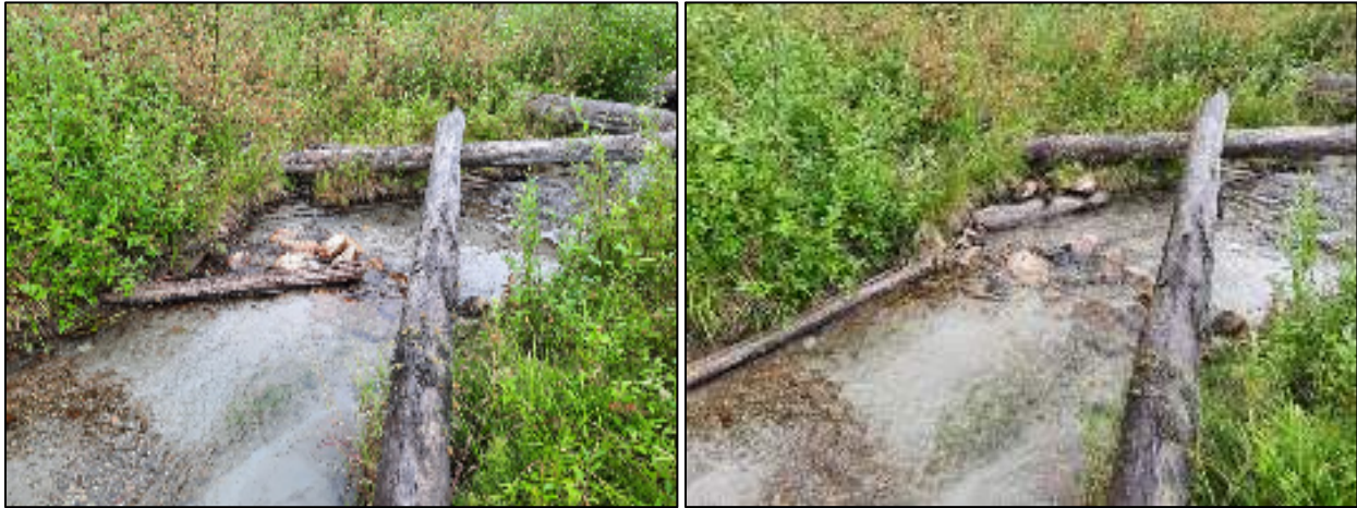
Figure 17. Restored riffle crest and bank protection near ALE-XS8, before (left) and after (right) repair. Flow is from left to right.
