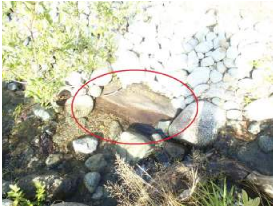
Figure 28. Exposed geotextile within the stream channel at ULL-ASTR04IM on August 24, 2020.
