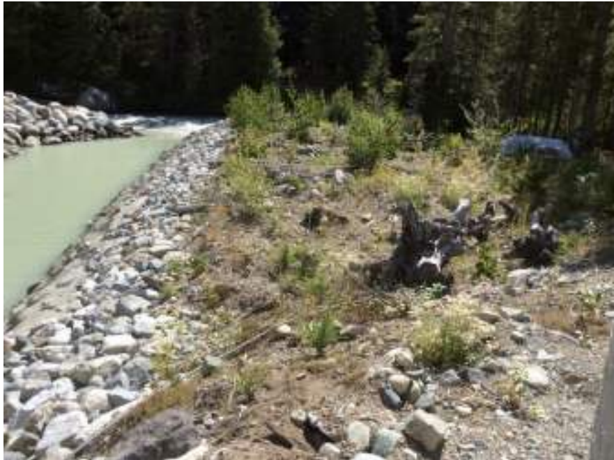
Figure 3. Representative site photo taken at 160° from BDR-PRM01 on September 1, 2020.
