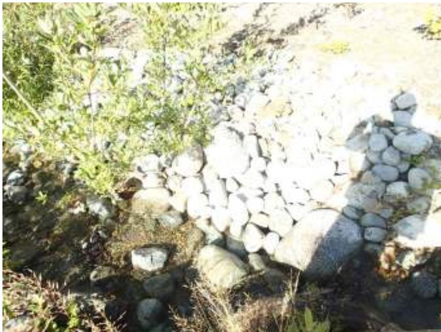
Figure 29. Location where geotextile had been exposed adjacent to the stream channel, after covering exposed section with cobble by hand, on August 24, 2020.
