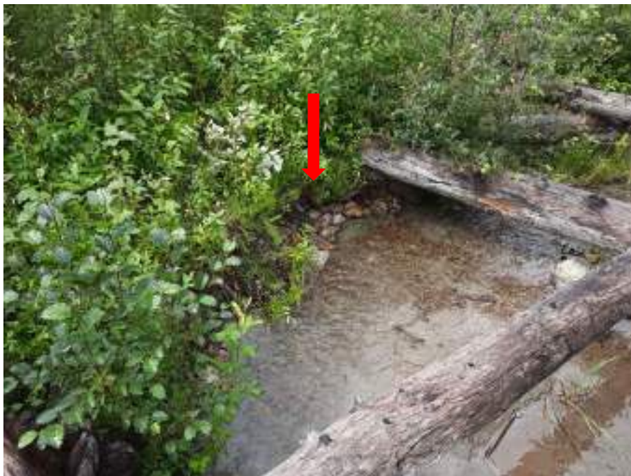
Figure 14. Bank stabilization repairs using cobble above ALE-XS7. Flow is from right to left.
