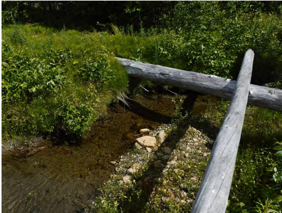
Figure 7. Bank erosion and channel down-cutting at ALE-XS5 requiring repair. Photo taken on June 20, 2019.
