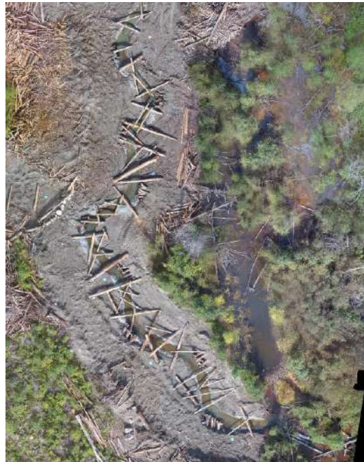
Figure 8. Aerial photo taken from the UAV showing the constructed channel for the Alena Creek FHEP on the left, and the retained beaver dam and pond on the right.
