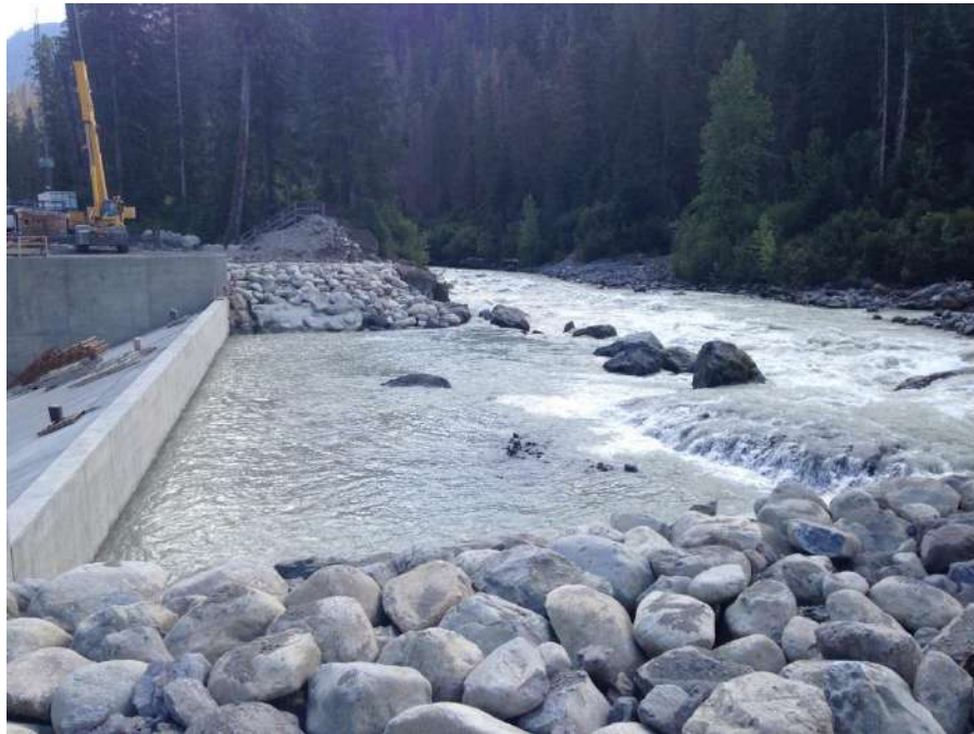
Figure 3. Upper Lillooet River HEF tailrace during the fall of 2016.
