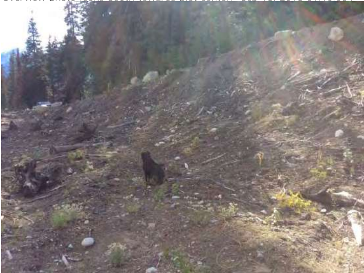
Card: Civil Works Stratum: Upper Lillooet Penstock/Plot: H/Comments Overview photo looks South towards plot center. Sep 18, 2018 01.15.06 P
