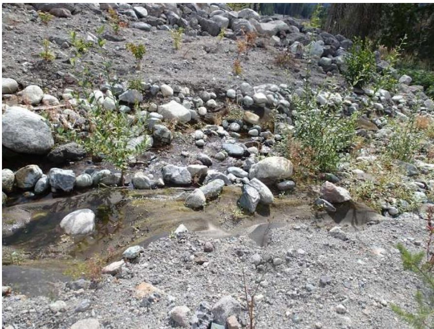
Figure 34. Exposed geotextile along ULL-ASTR04 on August 31, 2018.
