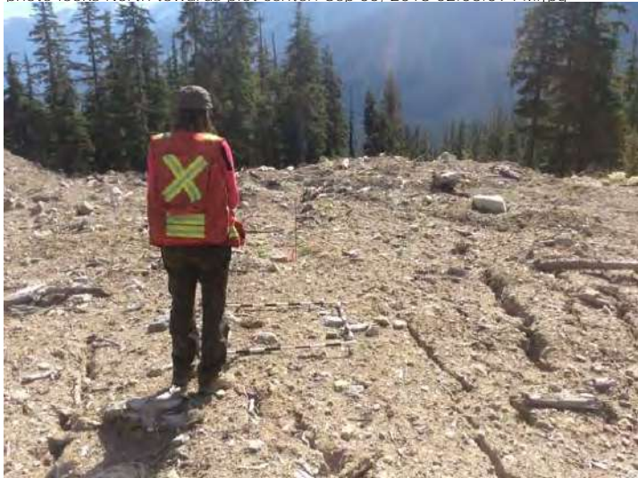
Card: Civil Works Stratum: Upper Spoil #8/Plot: 005/Comments Overview photo looks North towards plot center. Sep 05, 2018 02:03:09 PM.jpg
