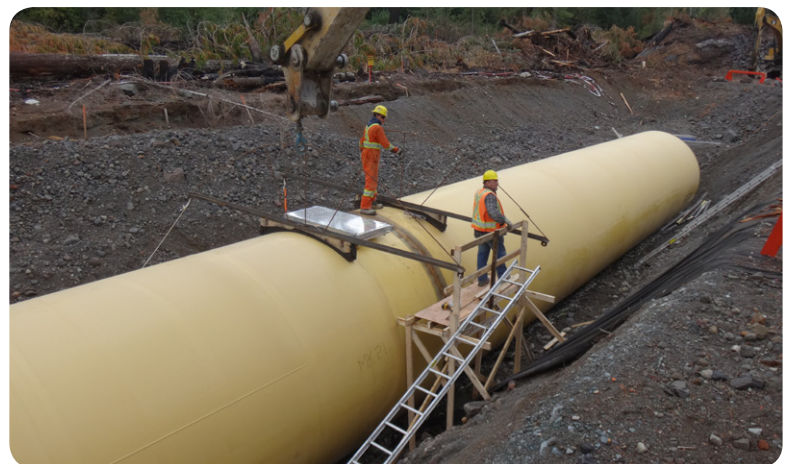
↑ September 3, 2015 - Upper Lillooet Penstock joint weld completed and crew setting up for corrosion protection.
