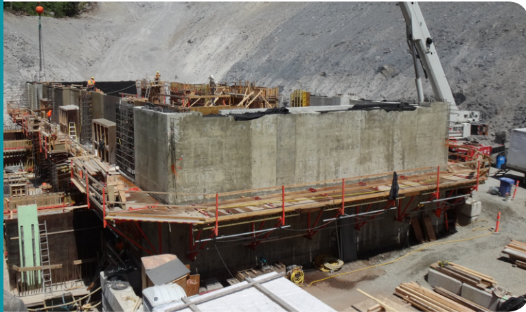
↑ June 6, 2015 - Upper Lillooet Powerhouse is 957.8 m 2 in size. Foundation consists of approximately 3,000 m 3 of concrete to date.
