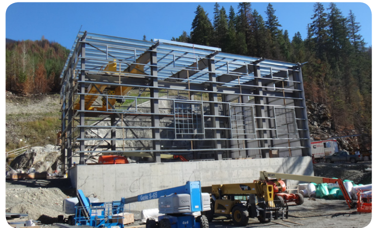
↑ September 11, 2015 - With just over 1,500 m 3 of concrete, the Boulder Powerhouse foundation is complete and the large steel superstructure is well underway. Two 42.5 tonne overhead cranes can be seen installed in the top of the structure. The Boulder Creek powerhouse is 792.6 m 2 in size.
