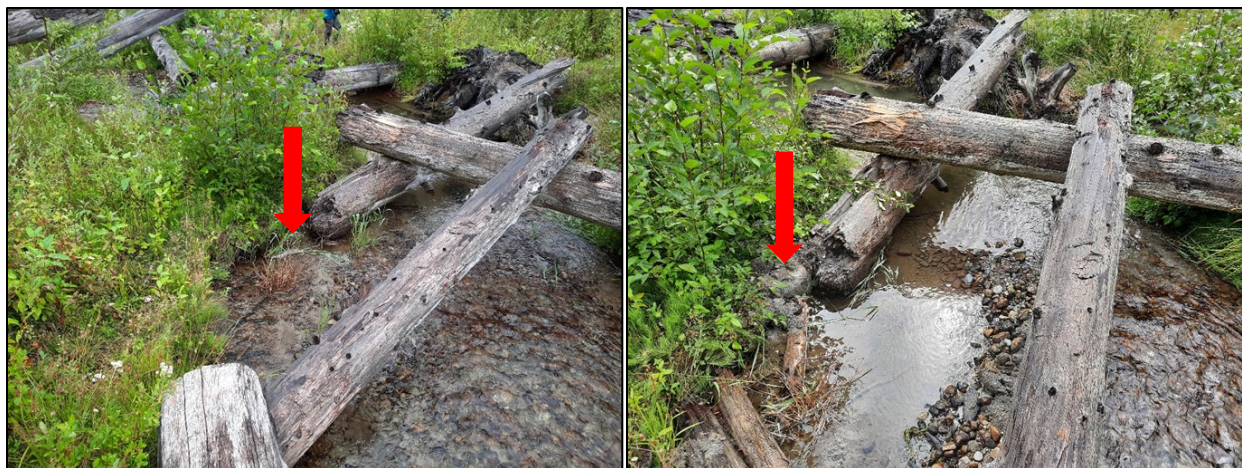
Figure 12. Bank erosion repair and gravel redistribution to create flow deflector near ALE-XS6, before (left) and after (right) repair. Flow is from bottom to top. Flow energy is concentrated away from eroding left bank and towards rootwads on river right.
