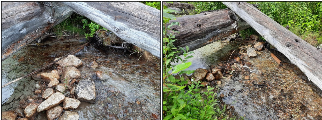
Figure 16. Restored riffle crest above ALE-XS7 before (left) and after (right) repair. Flow is from left to right.
