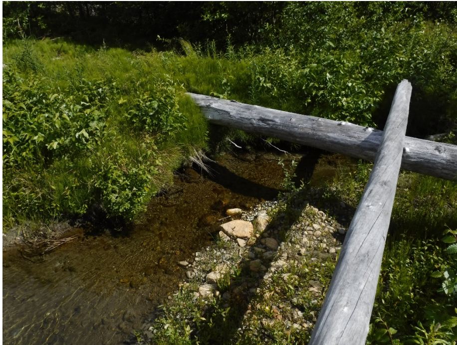
Figure 7. Bank erosion and channel down-cutting at ALE-XS5 requiring repair. Photo taken on June 20, 2019.
