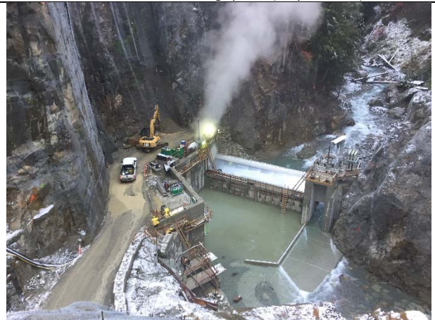
Photo 48 – Boulder Creek flowing through the sluice gate near completion of the intake structure (October 16, 2016)
