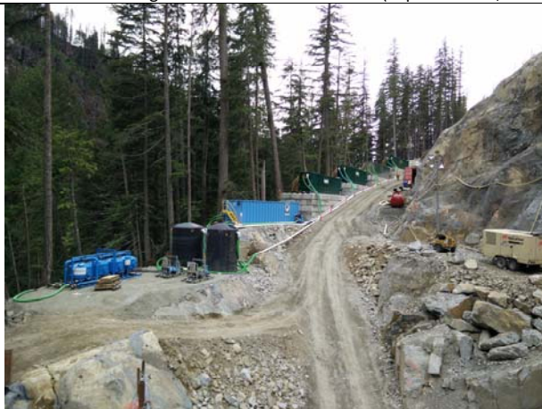
Photo 39 – Water treatment system (May 23, 2016)
