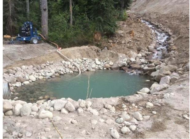
Photo 14 – Spring fed stream channelization and installation of a temporary access track and crossing to access the river right spoil area (June 12, 2014).
