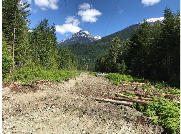
Photo 15 – Access road seasonal deactivation and reclamation (Segment 5 near the Lillooet River crossing; June 22, 2017).
