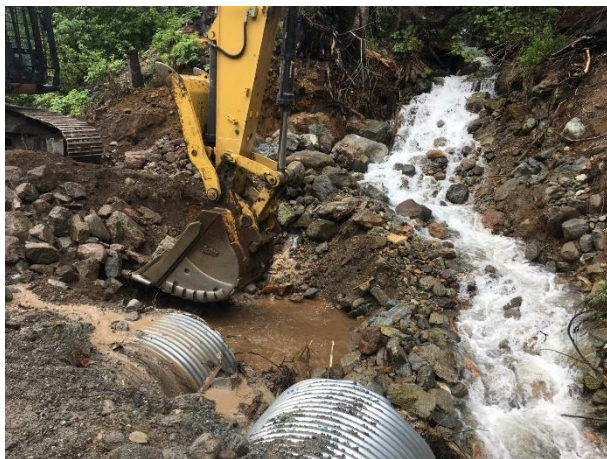
Photo 1 – Excavation and armouring of the KM41.2 culvert inlets with the majority of flow diverted (June 2, 2017).
