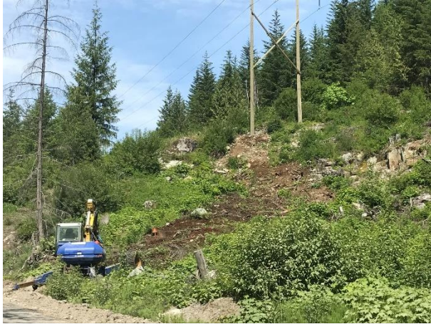
Photo 14 – Typical access road reclamation works in the North Zone (KM23 of the Lillooet River FSR; June 7, 2017).
