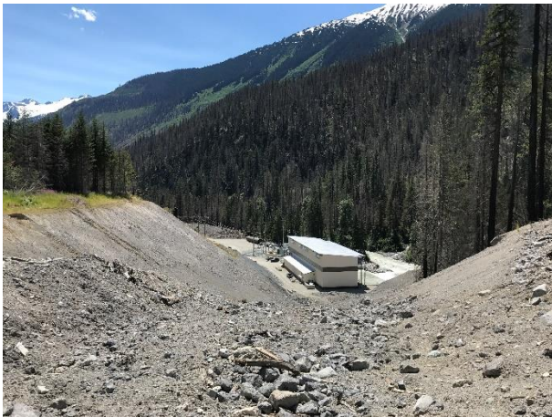
Photo 7 – Final condition of penstock leading to ULRHEF powerhouse. Alder seed has been spread (July 14, 2017).
