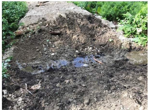
Photo 17 – Reclamation of the 185.1 access road in Segment 8 following culvert removal. Minimal flow infiltrated to ground following culvert removal (July 7, 2017).
