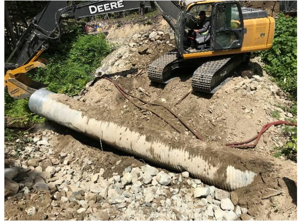
Photo 19 – Removal of the 600mm CSP culvert on the 184.1 access road in Segment 8 with bypass pumps in place (July 7, 2017).
