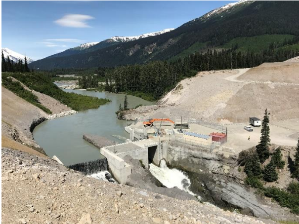
Photo 5 – Overview of the final condition of the ULRHEF intake river left area, slopes have been planted (July 14, 2017).
