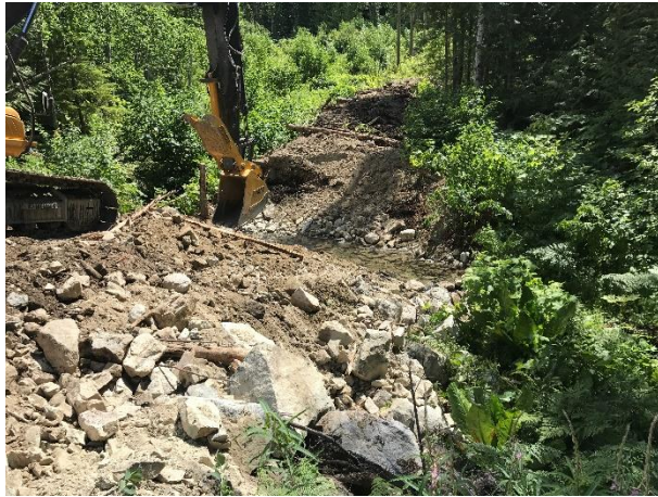
Photo 20 – Conditions ~30 minutes following the removal of the second culvert on the 184.1 access road in Segment 8 with bypass pumps removed and water flowing clear (July 7, 2017).
