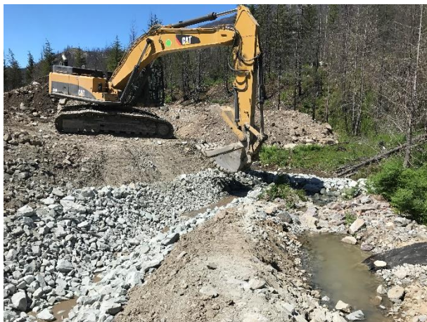
Photo 3 – Drainage tie-in at the completed BDRHEF powerhouse drainage ditch. All water infiltrated to ground and no surface water discharged offsite (June 22, 2017).
