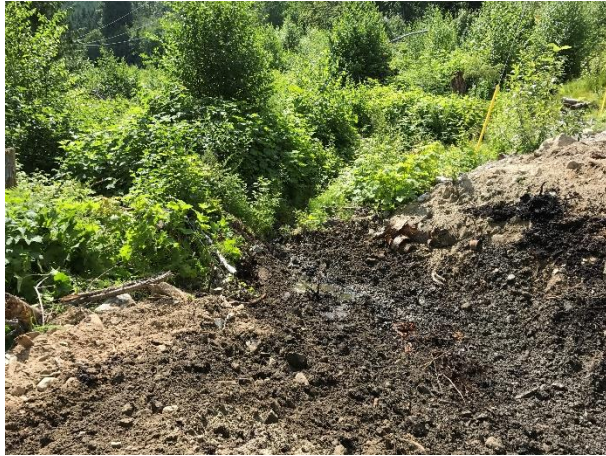
Photo 18 – Reclamation of the 184.1 access road in Segment 8 following removal of the smaller of the two culverts. Minimal flow infiltrated to ground following culvert removal (July 7, 2017).
