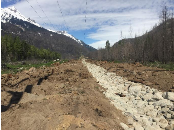
Photo 12 – Completed drainage and restoration under the transmission lines from BDRHEF powerhouse to the intake access road (May 22, 2017)
