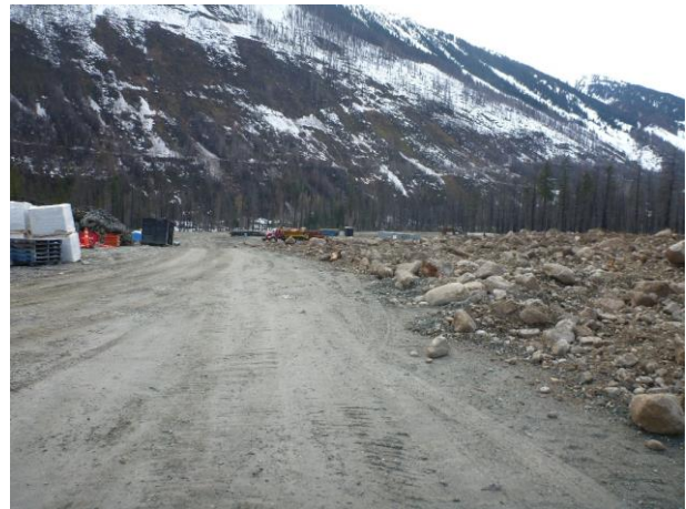
Photo 2 – Decompaction of the concrete batch plant site at the KM38 laydown (May 5, 2017).
