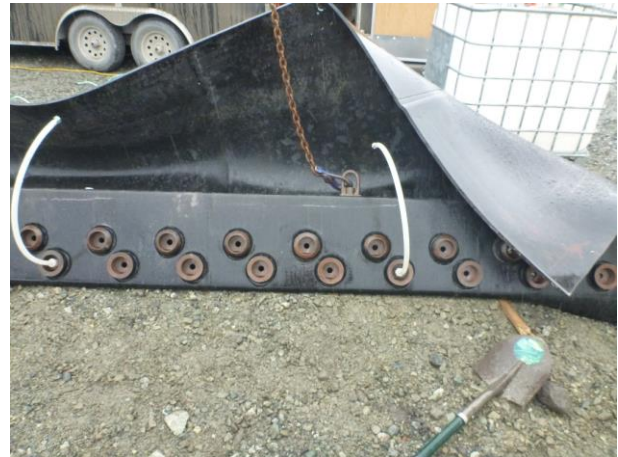
Photo 9 – Rubber Protective matting with angle iron and grouting ports to be installed on the ULRHEF sluiceway slab (May 5, 2017).
