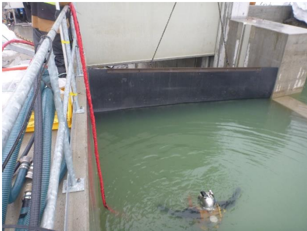
Photo 7 – Divers installing protective rubber matting on the upstream portion of the ULRHEF sluice way (April 13, 2017)
