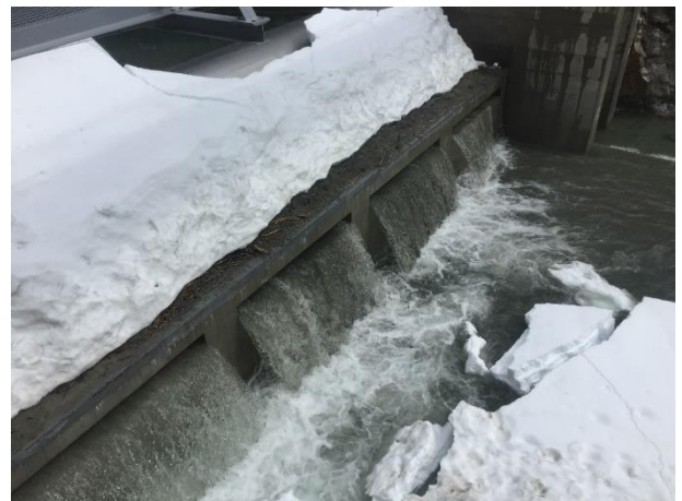
Photo 10 – Water and sand spilling out of the BDRHEF regulation channel (April 18, 2017)
