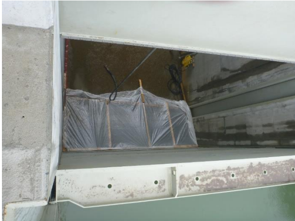
Photo 5 – Concrete works to repair a 2-meter section of the concrete on the downstream side of the ULRHEF sluice way (April 07, 2017)
