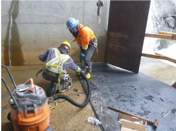
Photo 3 – Crews vacuum concrete dust while installing protective rubber matting on the downstream portion of the ULRHEF sluice way. (April 8, 2017)
