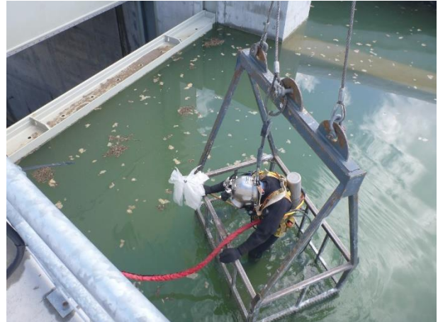
Photo 4 – Commercial divers inspecting the upstream portion of the ULRHEF sluice way slab (April 11, 2017)
