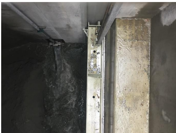
Photo 11 – Flushing sand out of the BDRHEF regulation chamber via the bypass gate (April 18, 2017)
