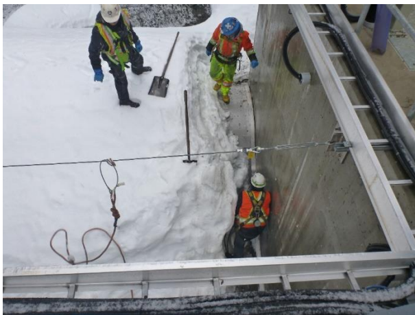
Photo 9 – CE patching concrete and caulking joints in the Coanda screen at the BDRHEF intake (April 14, 2017)
