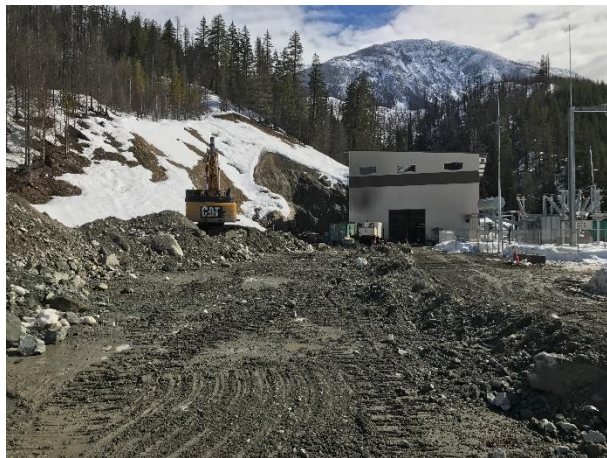
Photo 10 – CE began decommissioning the first three cells of the infiltration ponds (March 30, 2017).
