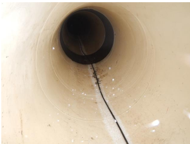
Photo 6 – Flushing water flowing down the BDRHEF steel tunnel liner (March 11, 2017).
