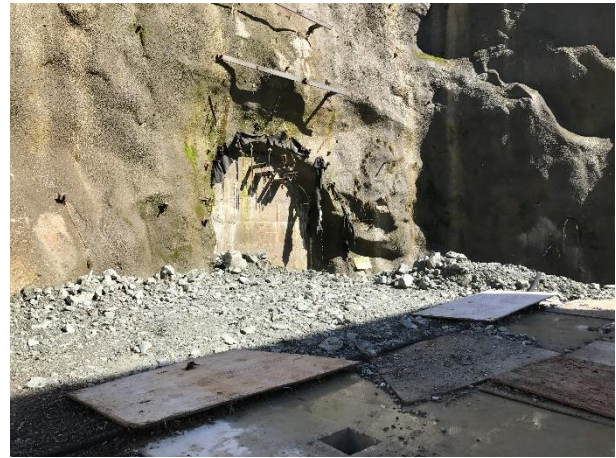
Photo 9 – BDRHEF tunnel portal. Cellular concrete and bifurcation concrete curing is occurring (March 30, 2017).
