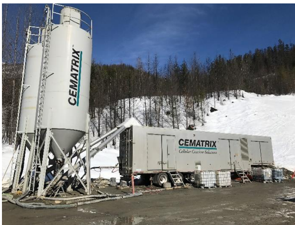
Photo 11 – Mobile concrete batch plant setup for cellular concrete production to encase the BDRHEF steel tunnel liner (February 23, 2017).
