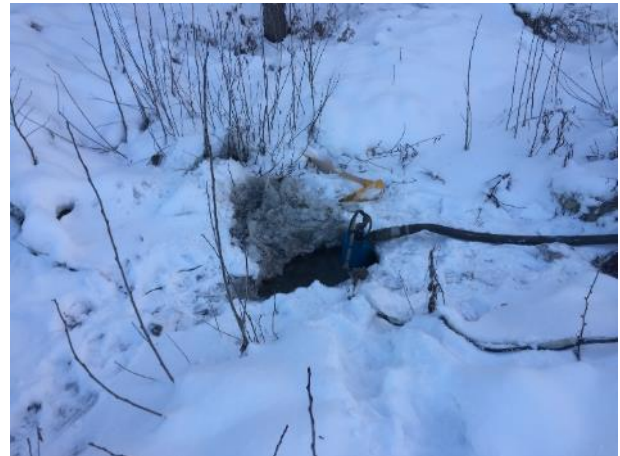
Photo 25 – Pump installed to capture seepage while installing the culvert at BDRHEF Spoil Pile (December 12, 2016).
