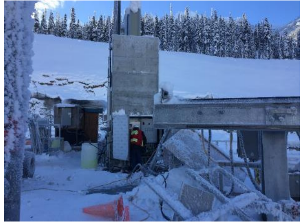
Photo 8 – Dry commissioning works at the ULRHEF Intake (December 15, 2016).
