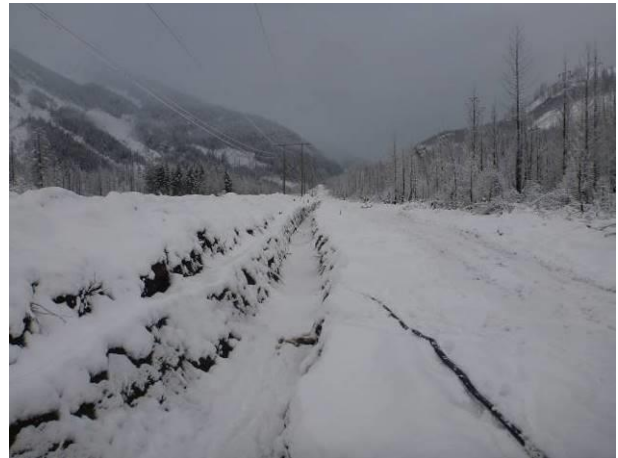
Photo 28 – Drainage channel excavated between the conduit access road and transmission line (November 30, 2016).
