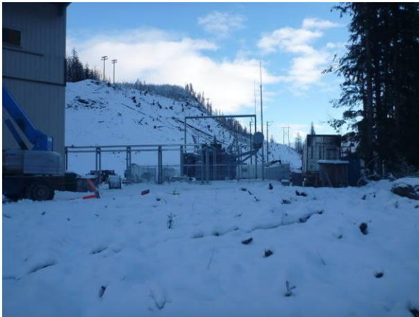
Photo 19 – ULRHEF switchyard (November 28, 2016)
