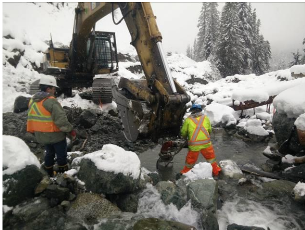
Photo 14 – Installation of a 6" pump to divert Truckwash Creek around the penstock over drain (December 2, 2016).
