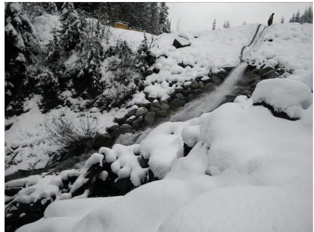
Photo 15 – Discharge of the 6" hose on to riprap downstream of the penstock over drain (December 2, 2016).
