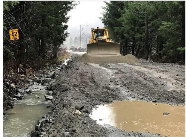
Photo 2 – Raising the elevation of the Lillooet River FSR between KM41.5 and 42.25 (November 22, 2016).
