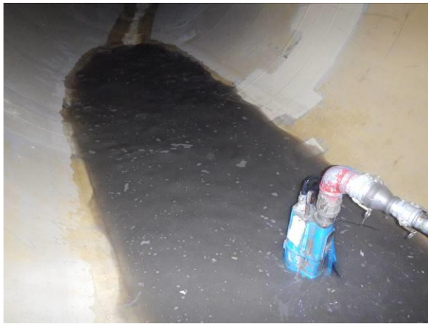
Photo 12 – Two-inch pump at the bottom of the penstock to capture flushing water to pump it into 1000L containers (November 25, 2016).
