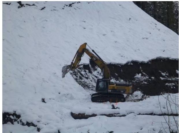
Photo 13 – Improper materials management while re-opening the Truckwash 2 access road (December 1, 2016).
