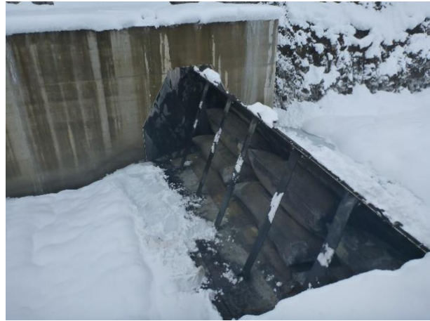
Photo 6 – Dry commissioning of the Obermeyer (November 30, 2016).
