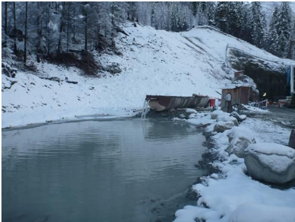
Photo 27 – BDRHEF lower tunnel portal sediment ponds (November 28, 2016).
