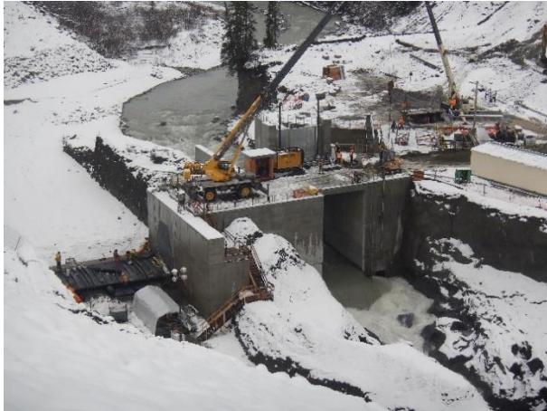
Photo 9 – Commissioning the ULRHEF intake gates (November 21, 2016).
