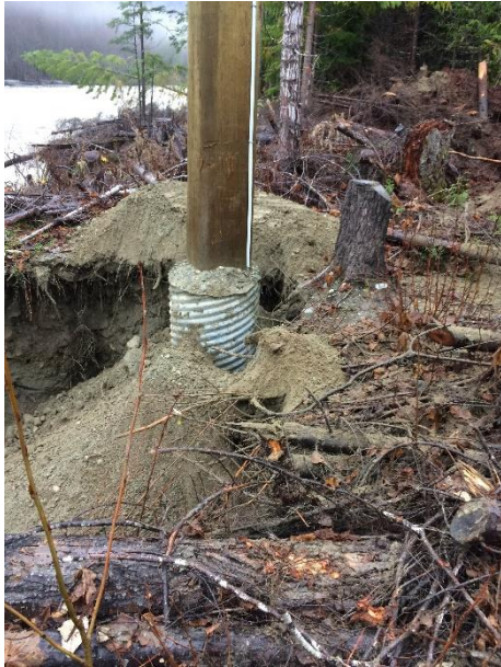
Photo 28 – Erosion from the November 9 flood at structure 139 (November 13, 2016).
