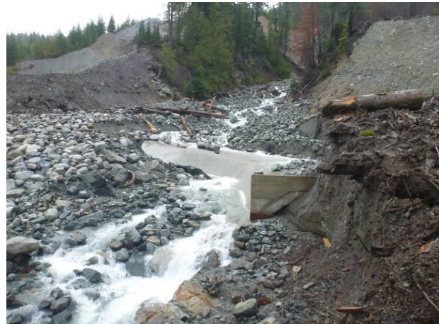
Photo 19 – Damage to the Truckwash Creek over-drain from the November 8 and 9 heavy rains (November 13, 2016).
