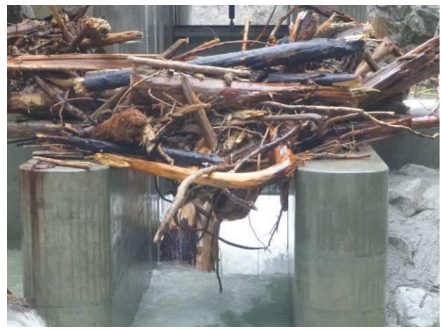
Photo 24 – Debris lodged on and in the BDRHEF sluice way (November 13, 2016).
