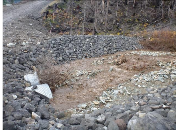
Photo 2 – Sediment pulse in ASTR-03 upon its diversion into its original channel post flood event (November 10, 2016).
