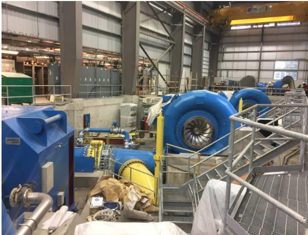
Photo 20 – Andritz mechanical works in the ULRHEF powerhouse (November 16, 2016).
