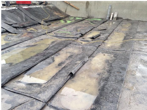
Photo 15 – Spilled sealant on the Obermeyer weir structure (November 18, 2016).
