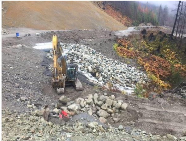
Photo 18 – Completion of the rip rap on the right bank of ASTR-03 (November 6, 2016).
