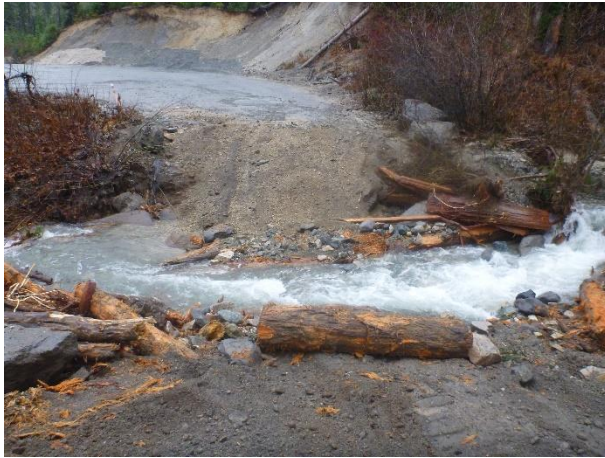
Photo 3 – Upstream KM48 woodbox culvert completely failed (i.e. washed out) in the heavy rain on November 8 and 9 (November 12, 2016).
