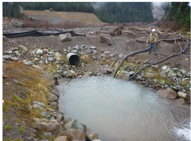
Photo 12 – Pumping the stream around the work area prior to removing the culvert (November 15, 2016).
