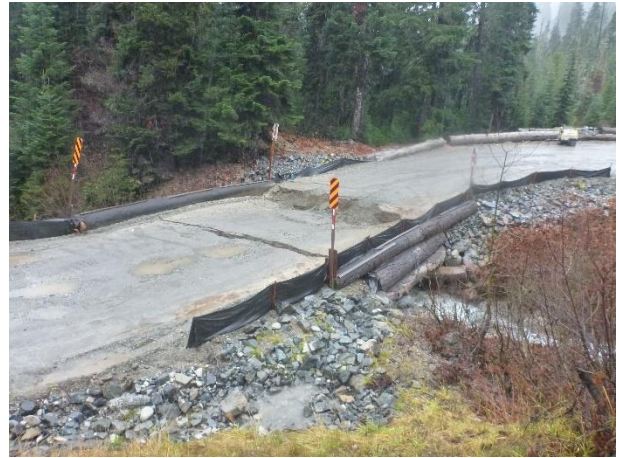
Photo 4 – Downstream KM48 woodbox culvert damaged in the November 8 and 9 heavy rains (November 11, 2016).
