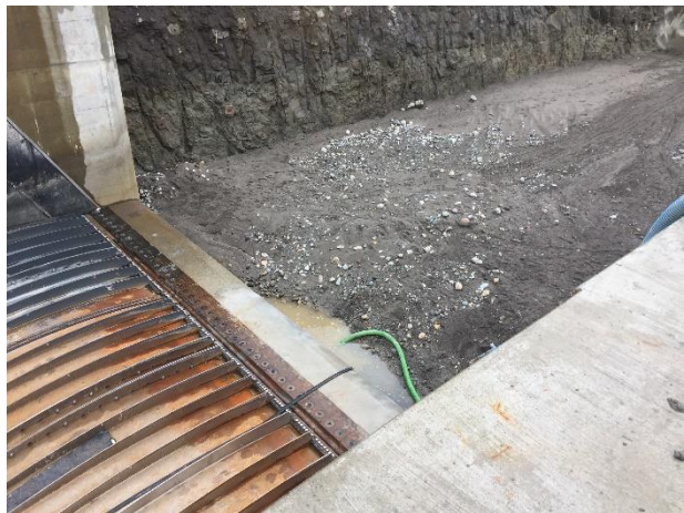
Photo 8 – Pumping high pH water above the Obermeyer channel to the water treatment system (October 31, 2016).
