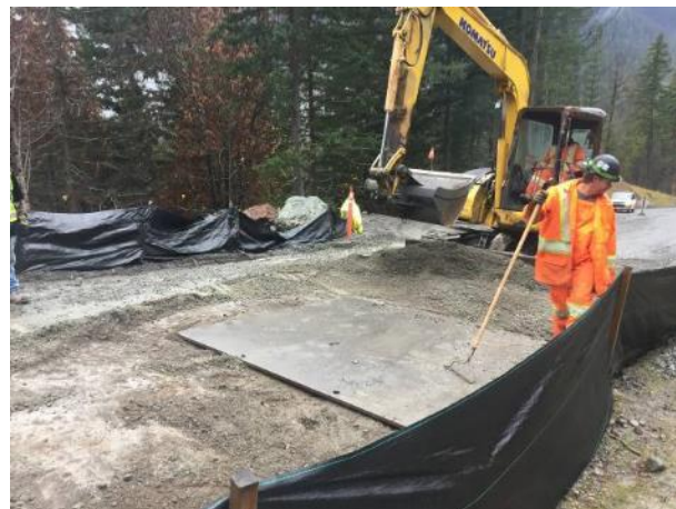
Photo 2 – Crews installing a steel plate to temporarily protect the KM43 culvert (October 29, 2016).
