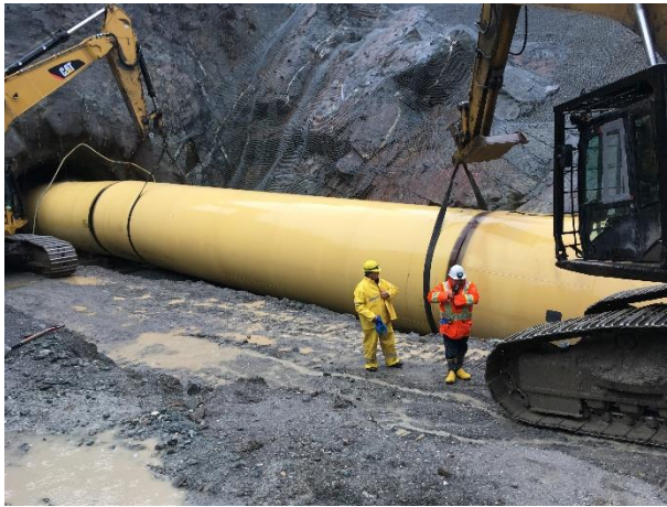
Photo 11 - Placement of the final penstock piece at the ULRHEF downstream tunnel portal (November 3, 2016).
