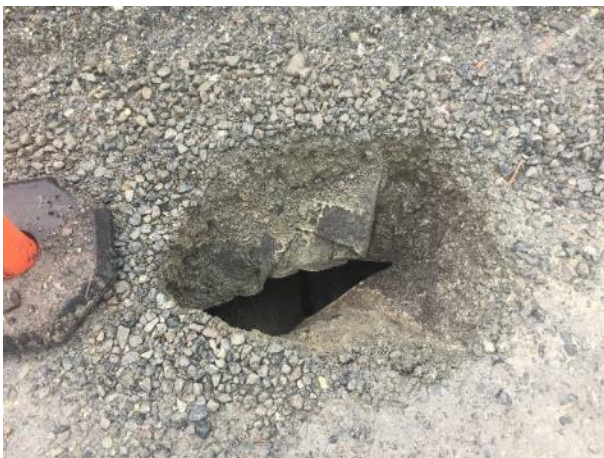
Photo 1 – A hole punctured in the culvert crossing the Lillooet River FSR at KM43 (October 29, 2016).
