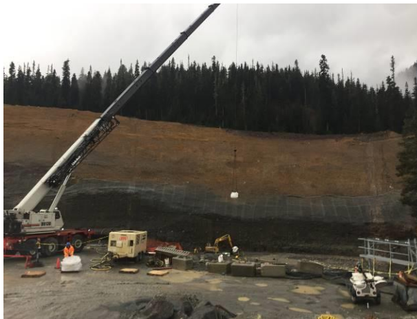
Photo 7 – Transport of shotcrete over the Lillooet River to the Obermeyer channel (October 29, 2016).
