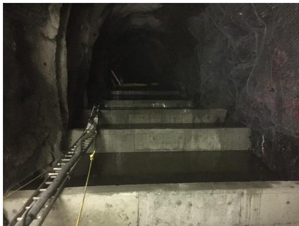
Photo 9 – ULRHEF rock trap filling with water from the tunnel flushing activities (October 30, 2016).
