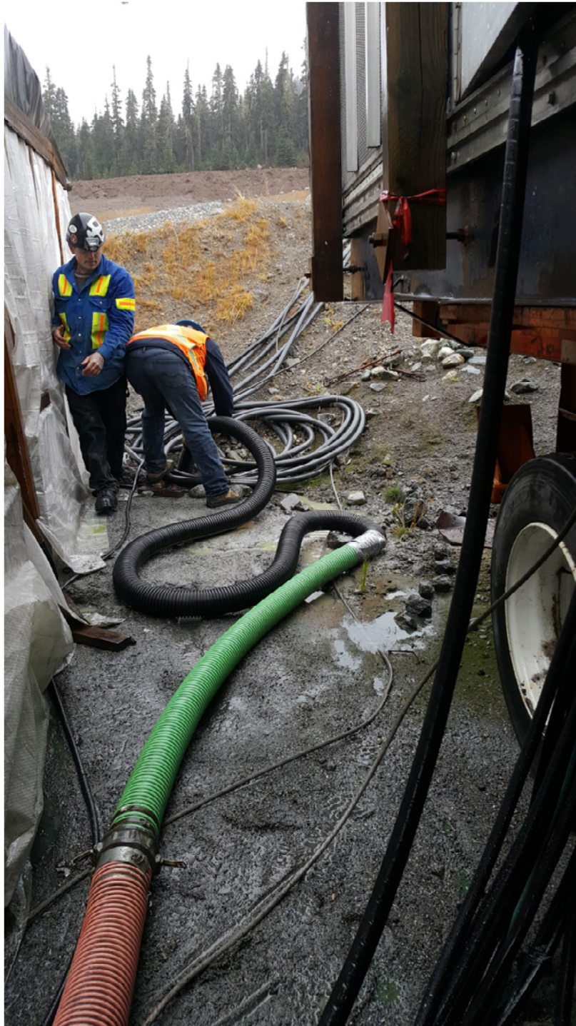
Figure 1: Vacuum truck removing contaminated water and sediment under generator tank
