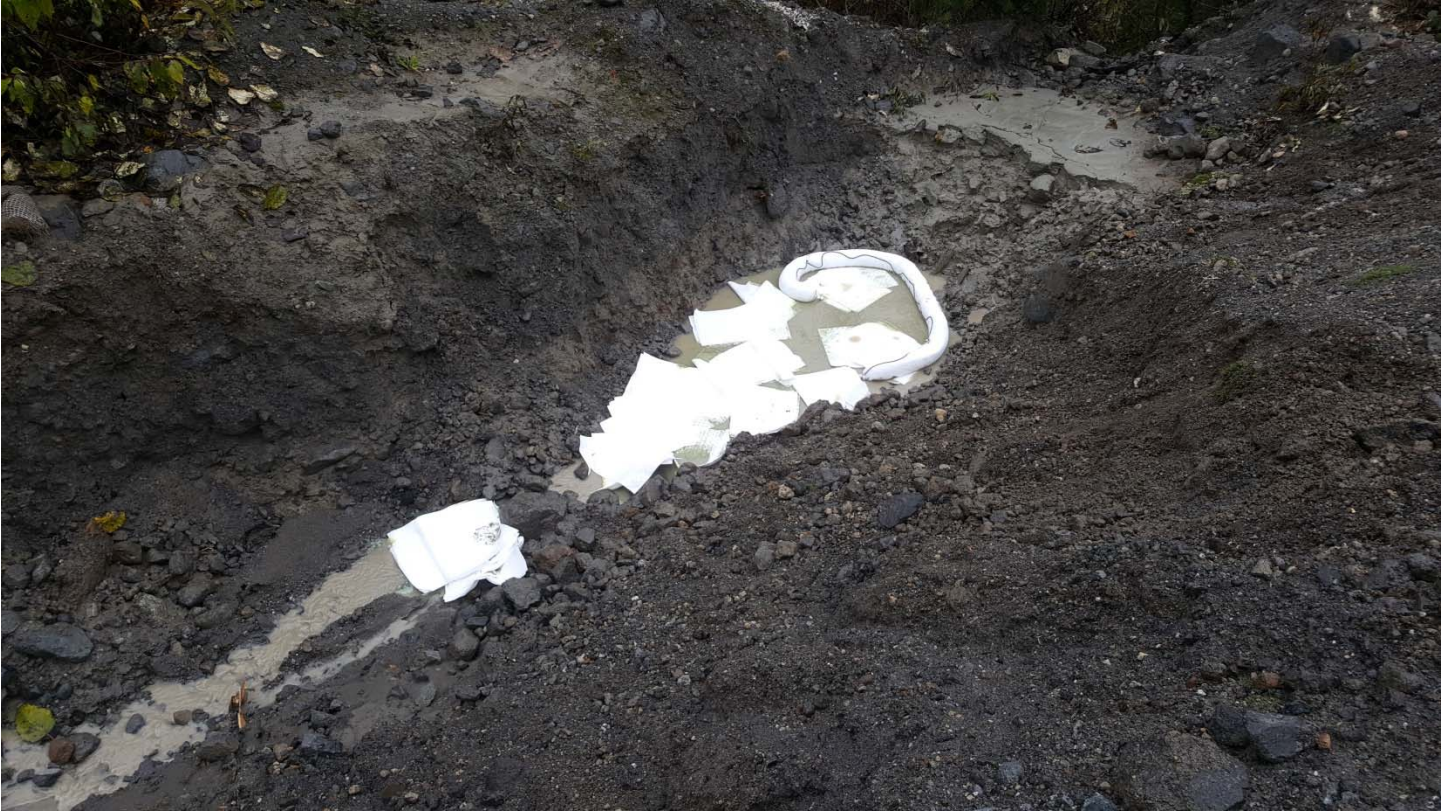
Figure 3: Spill booms and absorbent pads in sump
