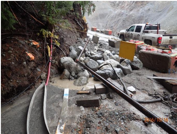
Photo 13 - Newly excavated infiltration pond and 2-inch pump at the small lower-tunnel portal lay down area (October 16, 2016).
