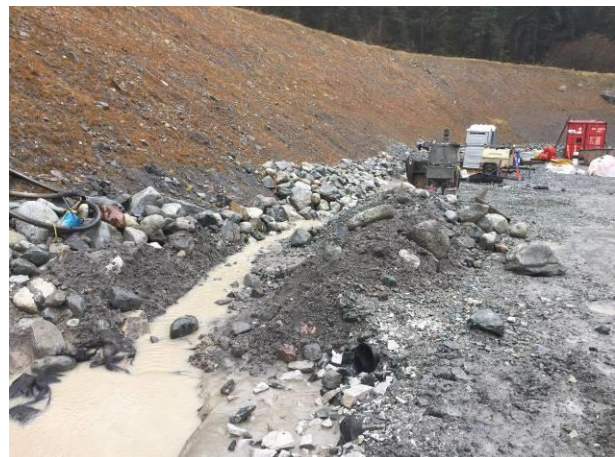
Photo 2 – Sediment laden water flowing towards KM49 bridge and pump sitting idle on slope (October 13, 2016).
