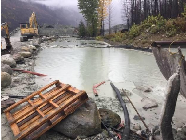
Photo 26 – BDRHEF lower-tunnel settling ponds (October 20, 2016).
