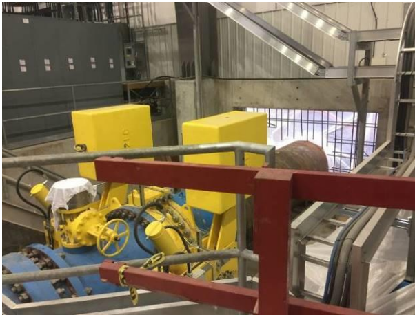
Photo 24 – Andritz mechanical works in the BDRHEF powerhouse (October 14, 2016).
