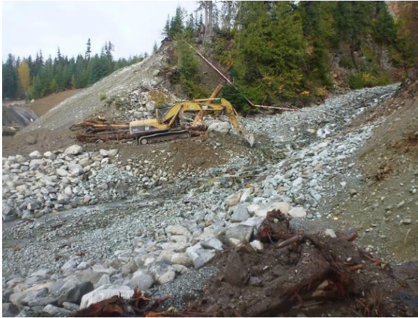
Photo 15 – Widening and armouring of the right bank of the Truckwash Creek over-drain (October 9, 2016).
