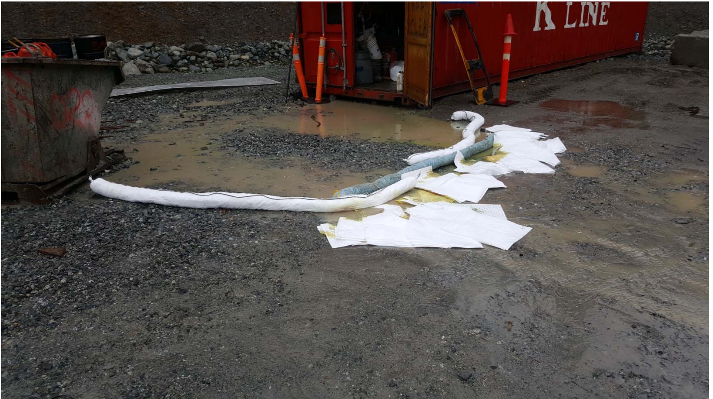
Figure 2: Spill booms and absorbent pads to stop migration of spill
