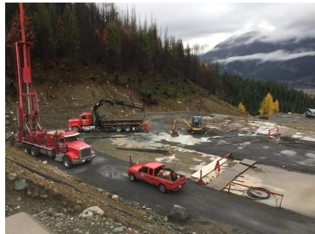
Photo 6 – Drilling for the permeant well on pad 2 of the construction camp (October 18, 2016).
