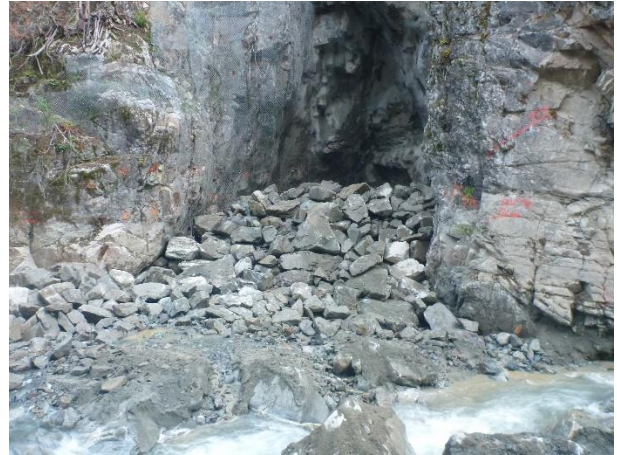
Photo 20 – Excavated material from the BDRHEF upstream cofferdam sealing the diversion tunnel (October 10, 2016).
