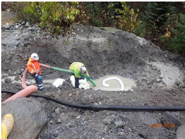
Photo 5 – Vacuum truck removing water and soil contaminated from diesel spill at KM48.5 (October 16, 2016).
