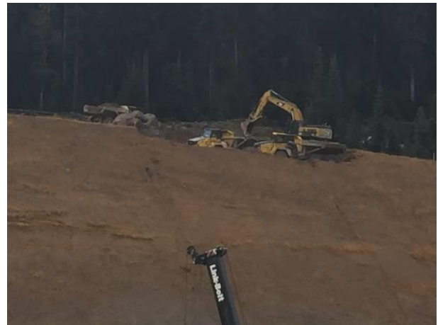
Photo 8 – Recontouring and reclamation of the slope on the right bank of the Lillooet River at the ULRHEF intake (October 22, 2016).
