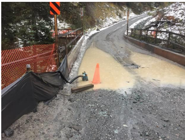
Photo 1 – Non-functioning pump installed on KM49 Bridge (October 13, 2016).
