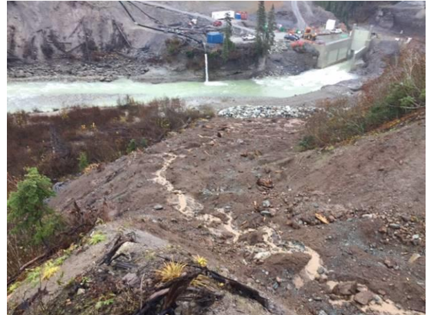
Photo 10 – Erosion on the old Obermeyer diversion channel access road (October 20, 2016).
