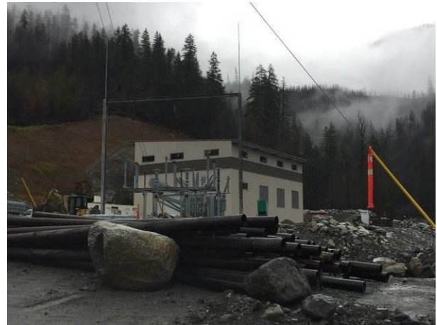
Photo 25 – BDRHEF switchyard (October 21, 2016).
