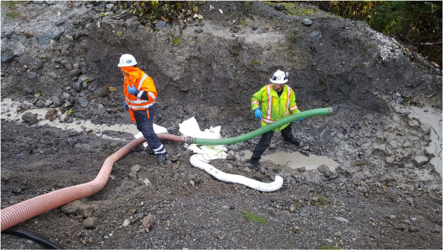
Figure 4: Vacuum truck removing contaminated water and sediment from sump
