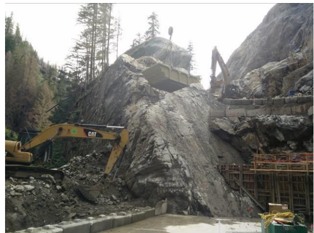
Photo 16 – Lowering the height of the downstream coffer dam to allow for rip rap placement (September 25, 2016).
