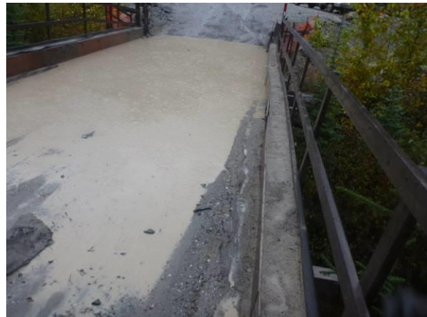
Photo 2 – Sediment laden water accumulating on Keyhole bridge (October 7, 2016).
