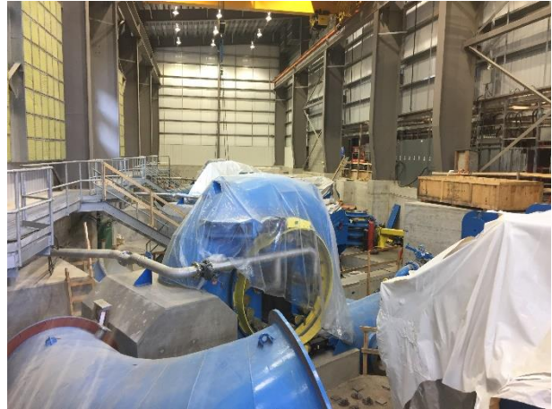
Photo 13 – ULRHEF powerhouse generators and turbines (September 30, 2016).
