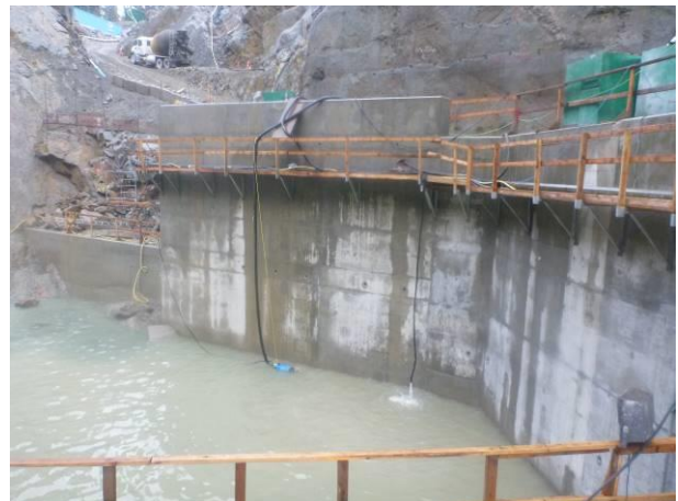
Photo 26 – CO 2 bubbler treating high pH water downstream of the Coanda spillway (October 7, 2016).
