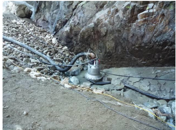
Photo 22 – Installation of sump to remove construction waste water to the active water treatment system (October 4, 2016).
