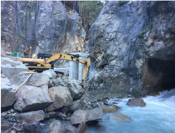
Photo 17 – Removal of the downstream coffer dam, all excavation occurred in the dry (September 29, 2016).
