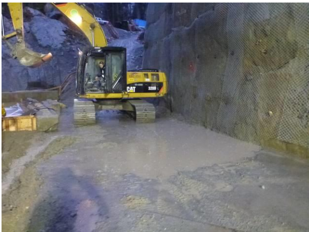
Photo 25 – Water with elevated turbidity and pH discharged to Boulder Creek (October 7, 2016).
