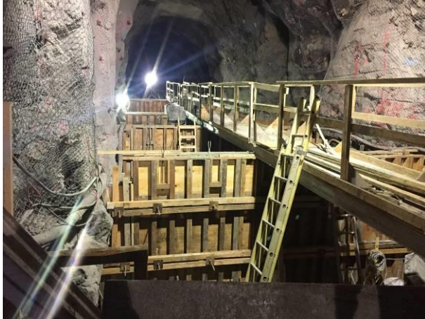
Photo 9 – Rebar, formwork, and concrete works on the lower-tunnel portal rock trap (September 30, 2016).
