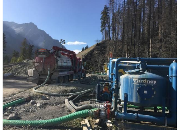
Photo 10 – Sediment removal and maintenance on the lower tunnel portal active water treatment system (September 30, 2016).
