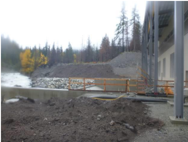
Photo 14 – Topsoil placement on the North and South sides of the ULRHEF tailrace (October 8, 2016).
