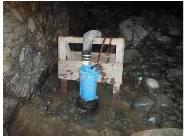
Photo 24 – pump installed in the diversion tunnel to capture construction waste water (October 5, 2016).
