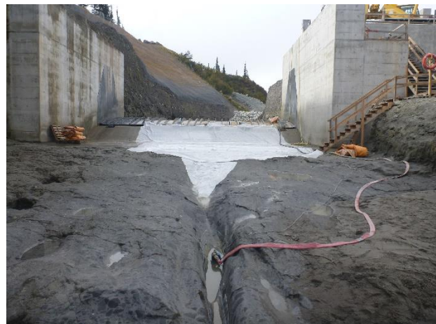
Photo 8 – Installation of a 2-inch pump to prevent high pH water from entering the Lillooet River (October 8, 2016).
