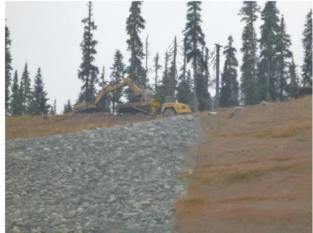
Photo 6 – Excavation of the final slope on the right bank of the ULRHEF intake structure (October 4, 2016).
