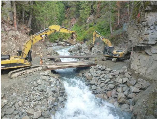
Photo 21 – Installation of a temporary bridge to access the diversion tunnel upstream of the BDRHEF intake structure (October 4, 2016).
