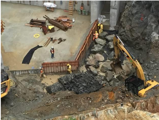
Photo 21 – Excavation of the BDRHEF downstream coffer dam, all works were conducted in the dry and above the high water mark (September 18, 2016).
