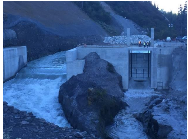
Photo 10 – Opening of the ULRHEF sluice gate (September 14, 2016).
