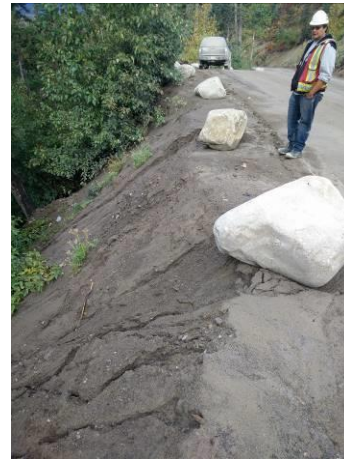
Photo 2 – Erosion on the downslope of the Lillooet River FSR at KM47 (September 20, 2016).
