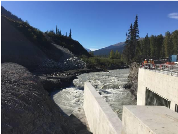
Photo 11 – Instream excavation to lower the elevation of the river channel and to fully divert the Lillooet River through the sluice way (September 15, 2016).
