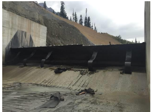
Photo 14 – Damage to the Obermeyer structure (September 16, 2016).
