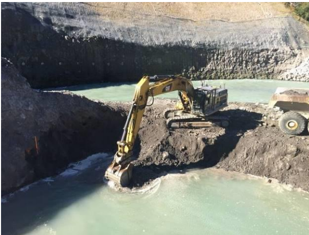
Photo 7 – Instream excavation once water levels were equal between the Lillooet River and the ULRHEF intake structure (September 12, 2016).
