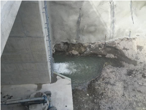
Photo 5 – Water leaking through the IFR gate at the ULRHEF intake structure (September 11, 2016).
