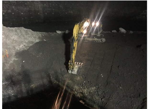
Photo 6 – Excavation of the ULRHEF upstream cofferdam to 300mm above river level on night shift (September 11, 2016).
