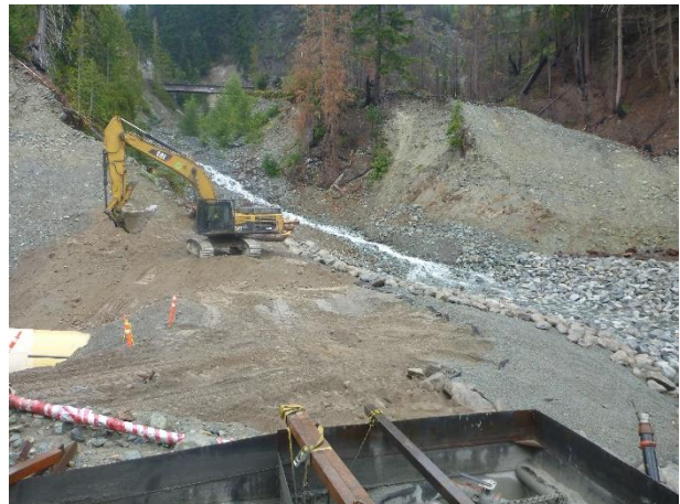
Photo 14 – Reclamation and landscape restoration on the west side of Truckwash Creek (September 7, 2016).
