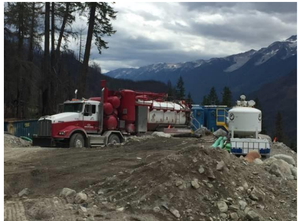
Photo 10 – Removal of deposited sediment from the Truckwash Creek active water treatment system (August 29, 2016).
