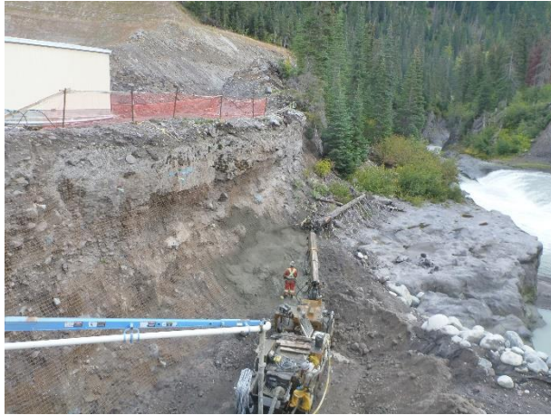
Photo 5 – Shotcrete application to stabilize the rock face below the ULRHEF intake control room (September 3, 2016).
