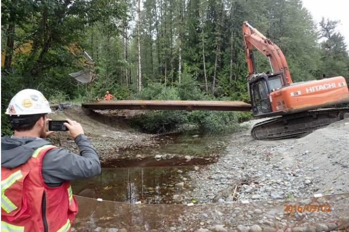
Photo 24 – Removal of the temporary bridge crossing installed to access pole structure 140 (September 2, 2016).
