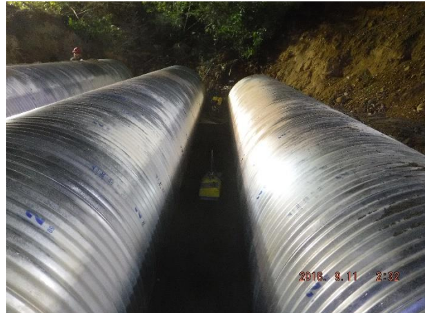
Photo 4 – Installation of the new 1600mm CSP for the KM41.2 stream crossing (September 10, 2016).
