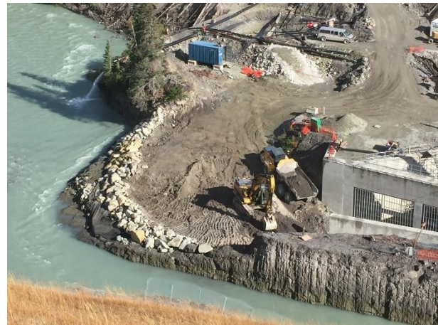
Photo 8 – Removal of a portion of the ULRHEF upstream cofferdam, in the dry (September 8, 2016).
