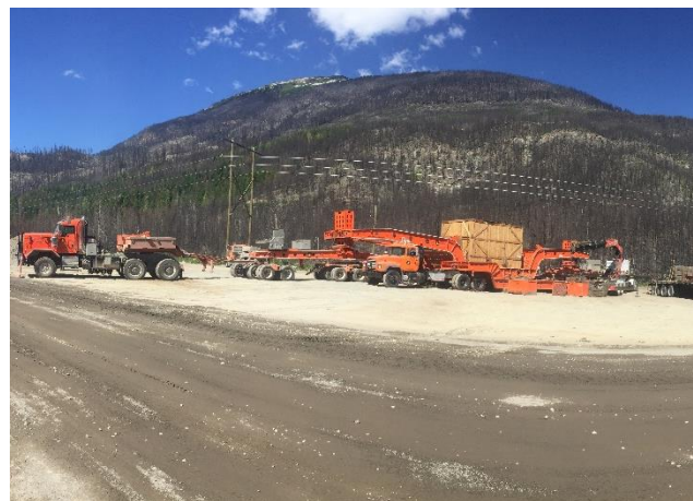
Photo 2 – Generator being transfer to a smaller specialized transport truck at the laydown at KM39 of the Lillooet River FSR (August 14, 2016).
