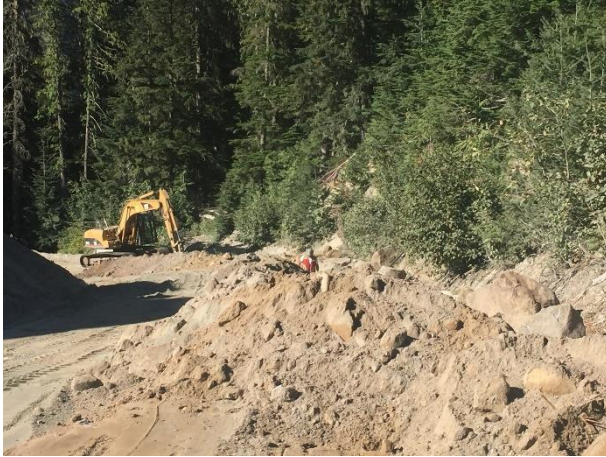
Photo 3 – Trenching and conduit installation along the ULRHEF lower tunnel portal access road (August 15, 2016).
