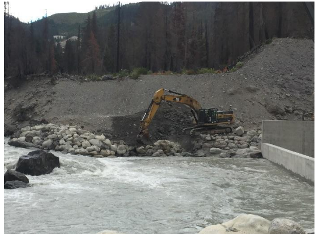
Photo 12 – Tailrace tie-in complete with continued rip-rap armoring placement in the dry (August 27, 2016).
