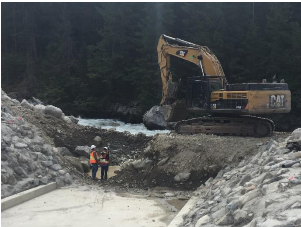
Photo 19 – Excavation and armouring of the upstream tailrace wall completed with an isolation berm in place (August 22, 2016).
