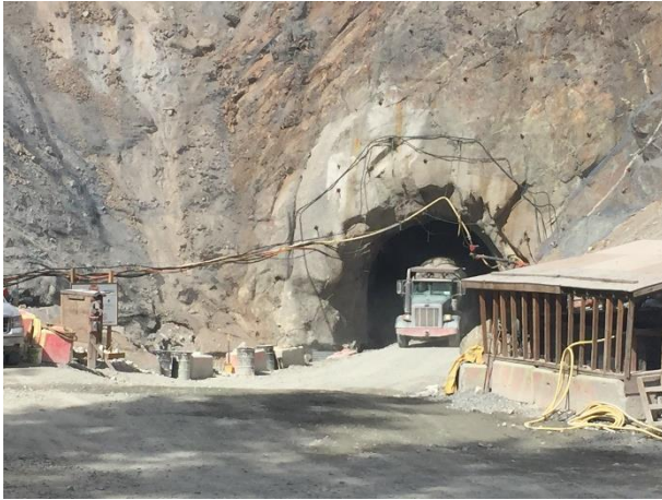
Photo 6 – Concrete truck backing into the lower tunnel to pour the tunnel floor liner at lower tunnel portal (August 22, 2016).
