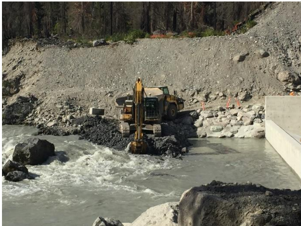
Photo 11 – Excavation of the final portion of the tailrace tie-in following 2 days of rock hammering bedrock (August 26, 2016).
