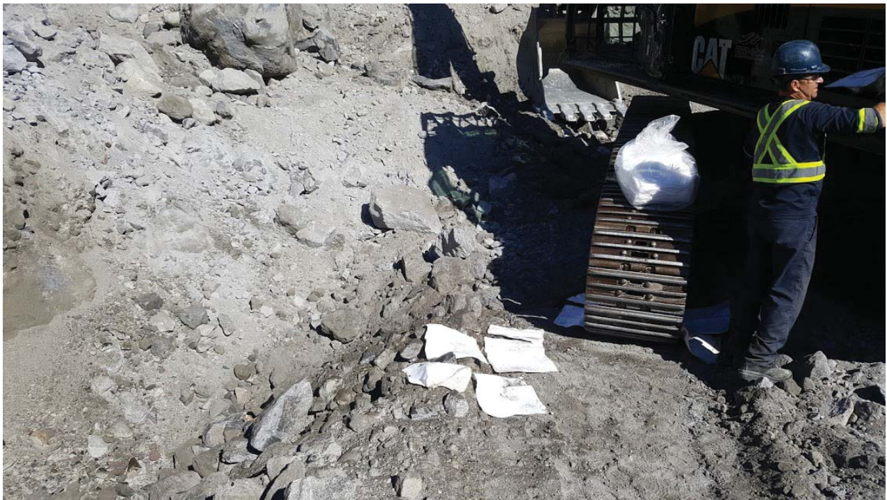
Picture 2 – Absorbent pads on the ground near the excavator
