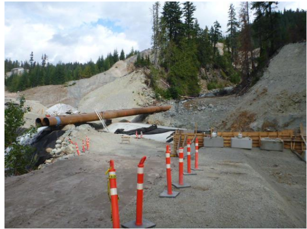
Photo 8 – Conditions at the Truckwash Creek crossing following the final pour for the protection slab/end wall (August 21, 2016).
