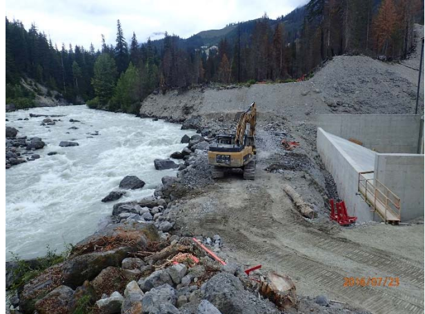
Photo 11 – Excavation for the ULRHEF tailrace, behind a natural earth berm, isolated from flowing water (July 23, 2016).
