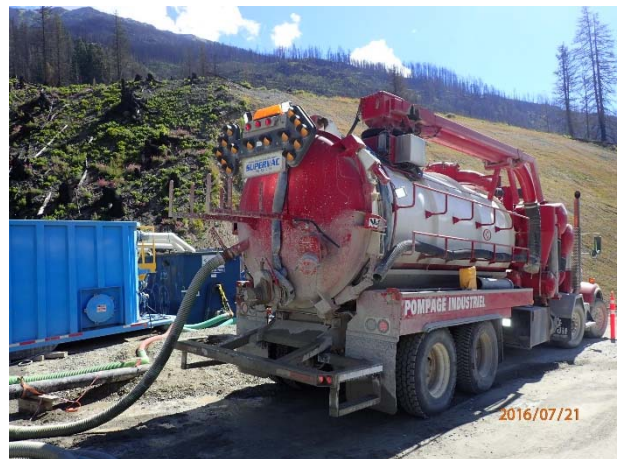
Photo 7 – Regular maintenance (sediment removal) from the primary ULRHEF lower tunnel portal active water treatment system (July 21, 2016).
