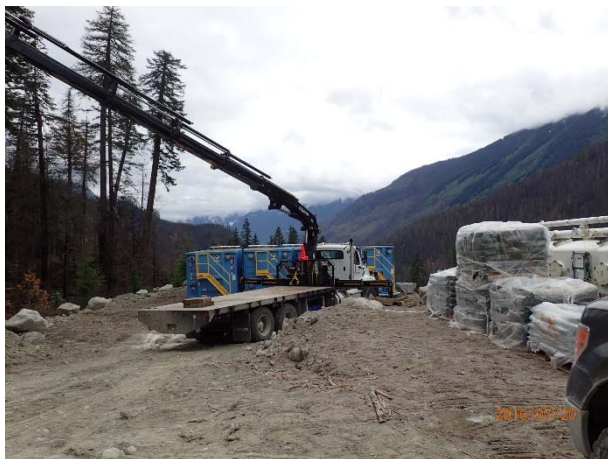
Photo 6 – Installation of second active water treatment system at the ULRHEF lower tunnel portal (July 20, 2016).
