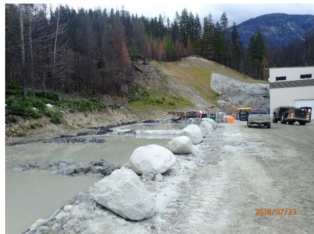
Photo 18 – BDRHEF downstream portal settling ponds and CO 2 injection box (July 23, 2016).
