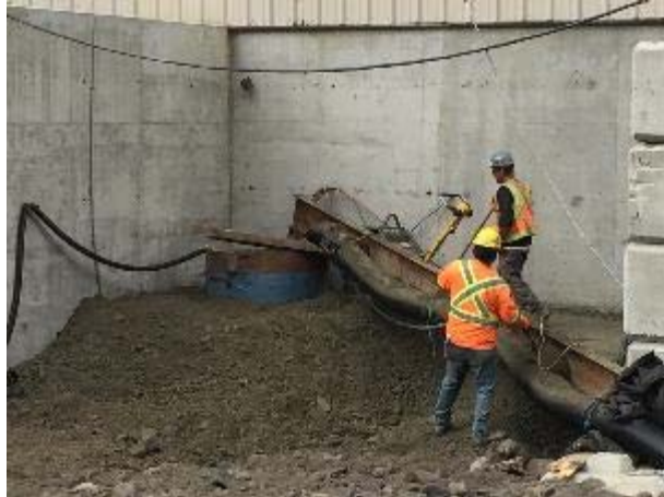
Photo 10 – Completion and backfill around the new clean water sump at the ULRHEF powerhouse (July 19, 2016).
