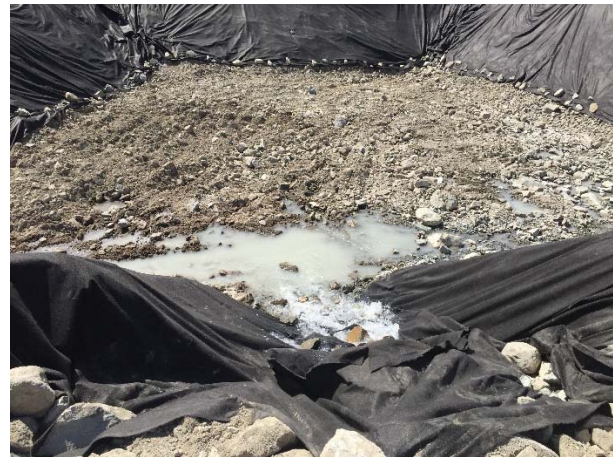
Photo 20 – Water infiltrating into the ground within the newly constructed settling/infiltration pond (July 27, 2016).
