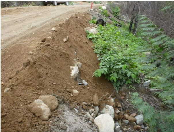
Photo 17 – Culvert outlet blocked by excess conduit trenching material at KM0.5 of the BDRHEF intake access road (August 8, 2016).
