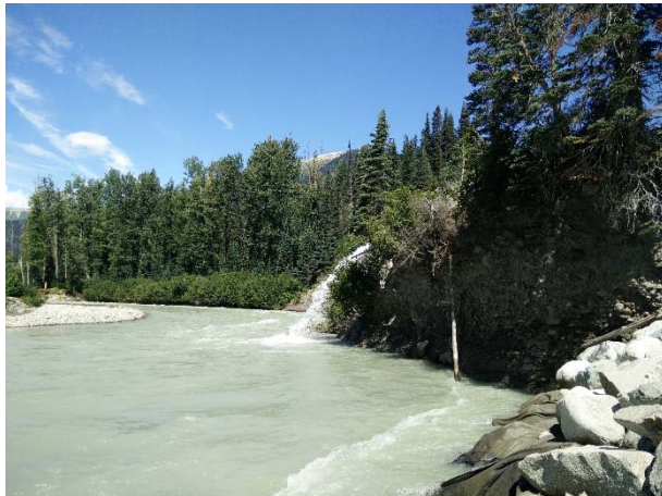
Photo 6 – Discharge of ULRHEF upper active water treatment system relocated upstream of the cofferdam (August 6, 2016).
