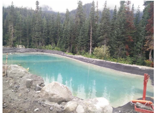
Photo 7 - ULRHEF upper tunnel water treatment system, pond 7 (August 9, 2016).
