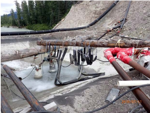
Photo 9 – New discharge water line from the concrete lined sump at ULRHEF (July 11, 2016).
