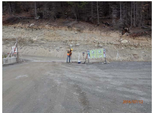
Photo 2 – Removal of the gap between the electric mat and electric fence at pad 3 entrance to the construction camp (July 12, 2016).
