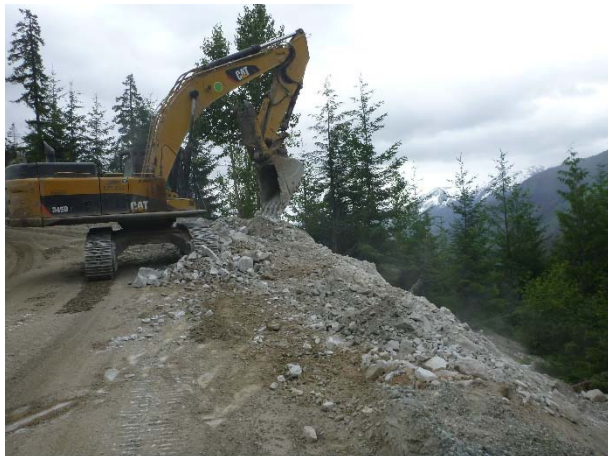
Photo 3 – Clean-up of material dumped at KM45.3 of the Lillooet River FSR (July 4, 2016).
