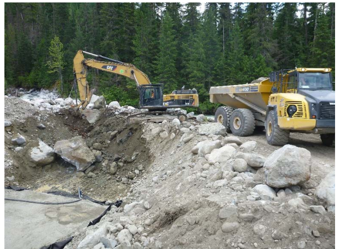
Photo 20 – Excavation for the second stage of the BDRHEF tailrace concrete works (July 16, 2016).
