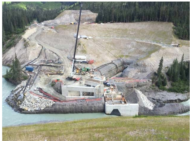
Photo 6 – ULRHEF intake (July 5, 2016).
