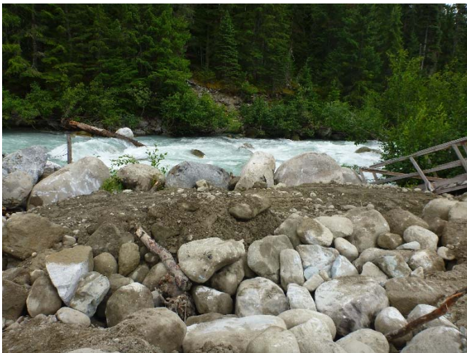
Photo 19 – Berm for constructed behind the high water mark at BDRHEF tailrace (July 15, 2016).
