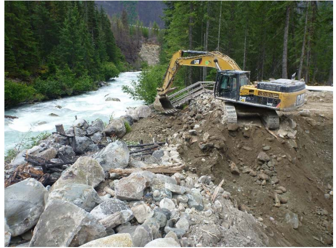
Photo 18 – Placement of large boulders for debris berm along the high water mark of Boulder Creek (July 15, 2016).
