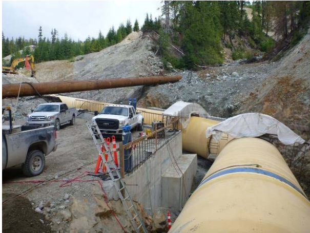
Photo 11 – Welding and coating works on the ULRHEF penstock through the Truckwash Creek diversion (July 15, 2016).
