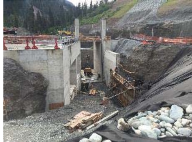
Photo 4 – Rebar, formwork, and concrete works at the ULRHEF sluiceway and intake (June 14, 2016).
