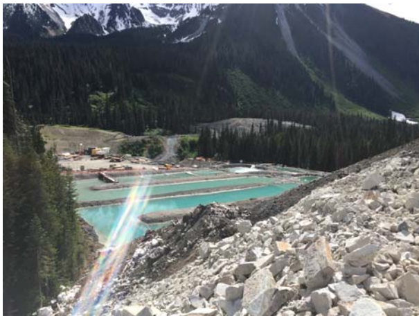
Photo 5 – ULRHEF water treatment ponds (June 15, 2016).
