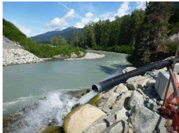
Photo 6 – Discharge of ULRHEF intake water treatment system (June 18, 2016).
