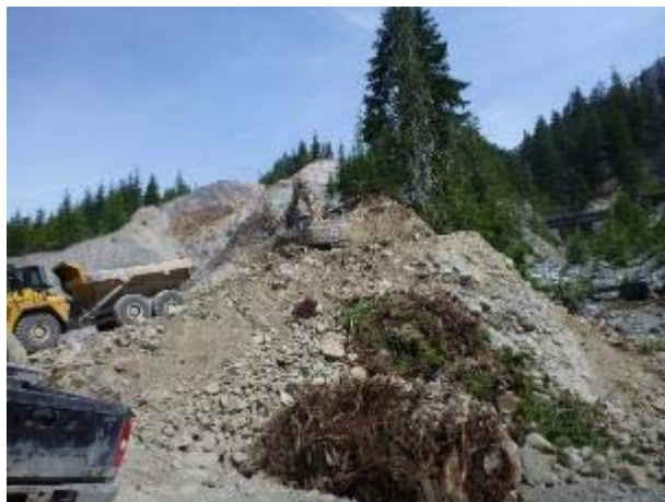
Photo 8 – Excavation of the Truckwash Creek mountain goat migration corridor audio-visual barrier (June 7, 2016).
