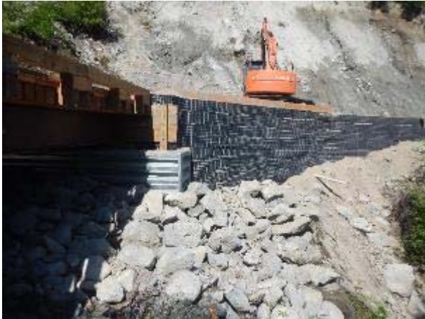
Photo 20 – Finalizing the installation of the mechanically stabilized wall on the west abutment of bridge 272a (June 7, 2016).
