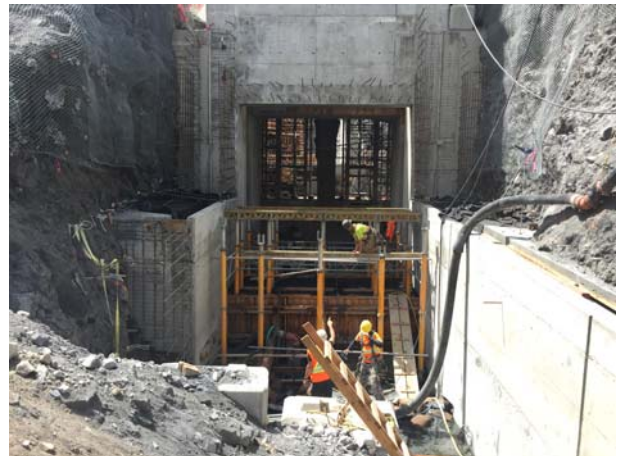
Photo 3 – Works on the transition between the intake structure and the BEBO wall (May 29, 2016).
