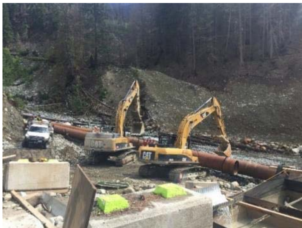
Photo 9 – Installation of steel bypass pipes prior to the Truckwash Creek diversion (June 02, 2016).
