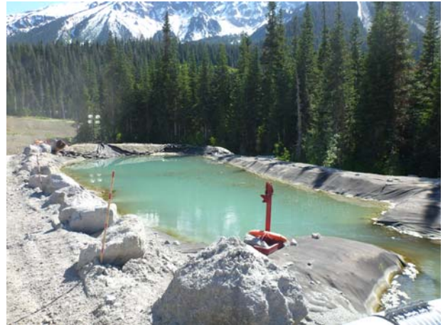
Photo 5 – Pond 6 and 7 of ULRHEF intake water treatment system (June 04, 2016).
