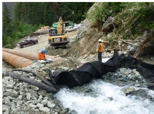
Photo 12 – Inlet of Truckwash Creek temporary bypass pipes following the diversion works (June 03, 2016).
