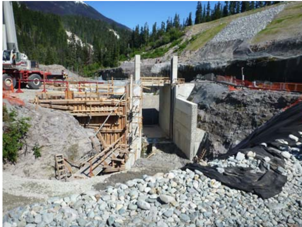
Photo 4 – Rebar, formwork, and concrete works at the ULRHEF sluiceway and intake (June 04, 2016).
