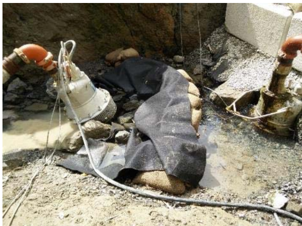
Photo 13 – Division of clean water sump at ULRHEF tailrace (May 23, 2016).
