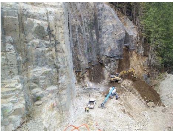
Photo 19 – Consolidation and stabilization of Boulder Intake rock face, and excavation for concrete works (May 23, 2016).
