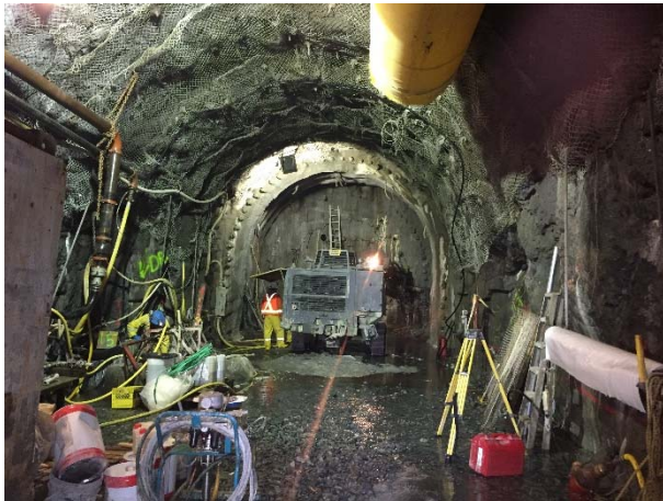
Photo 5 – Drilling probe holes into the grouting tunnel face prior to beginning mechanical excavation (May 10, 2016).
