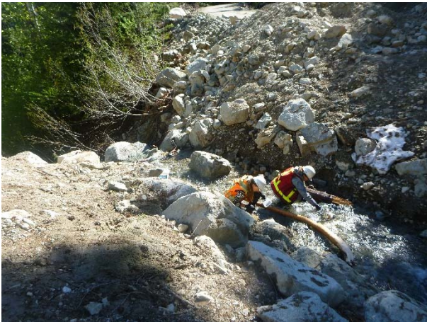
Photo 25 – Precautionary CTF salvage in stream 272a prior to performing a one-time crossing with an excavator equipped with bio-oil (Segment 11; May 10, 2016).
