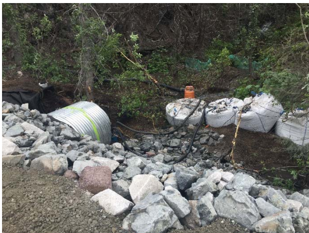
Photo 3 – ASTR-04 culvert installed outside of the natural channel alignment (May 18, 2016).
