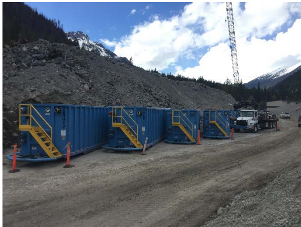
Photo 15 – Installation of the water treatment system designed to treat water from the ULRHEF tailrace excavation (May 12, 2016).
