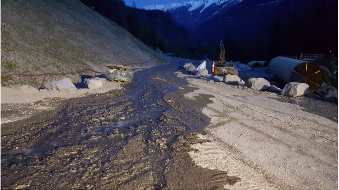
3. Water flowing down Truckwash access road
