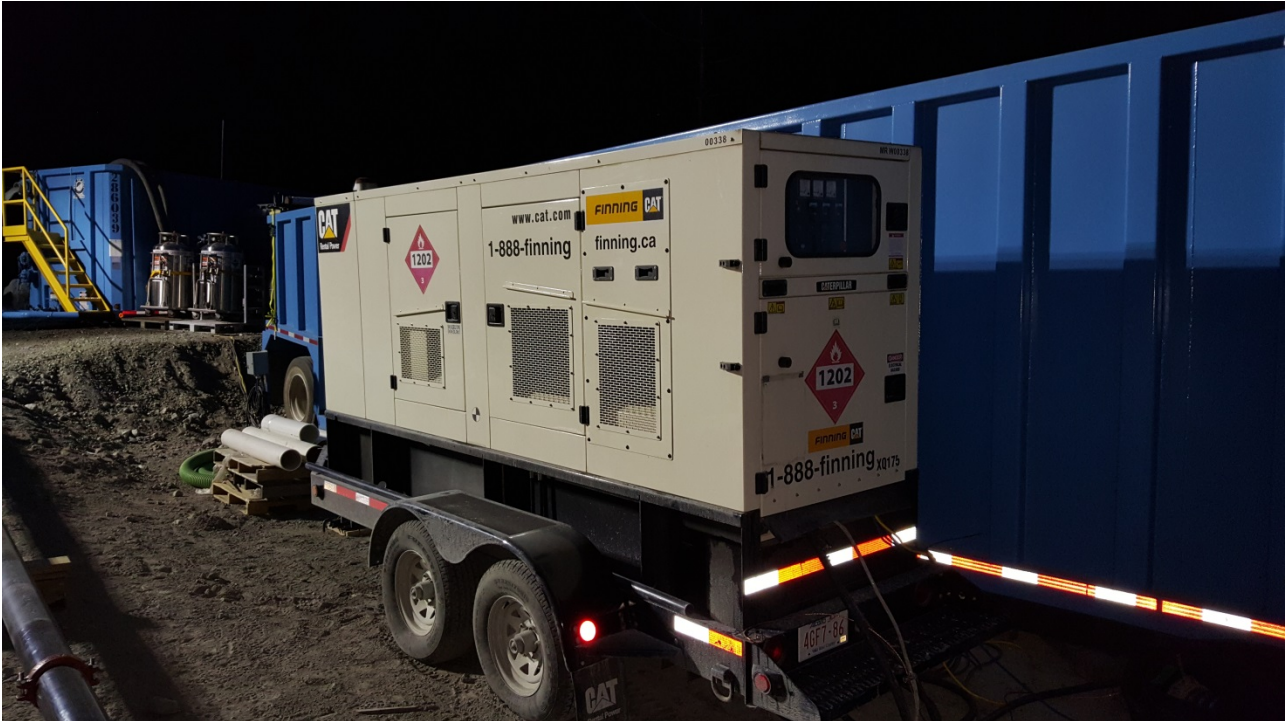
4. The generator at fault
