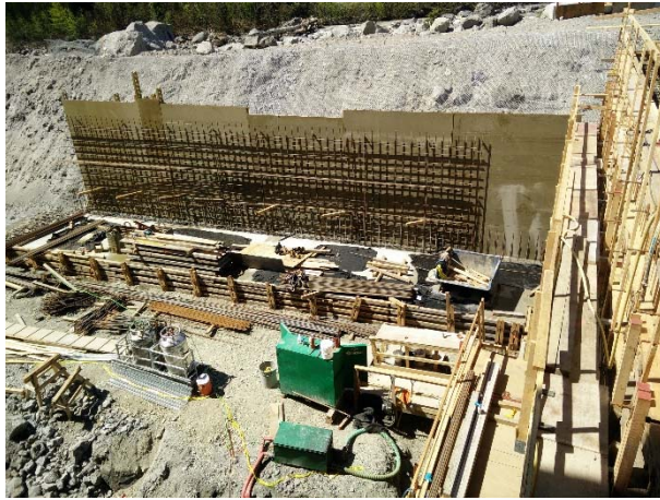
Photo 13– Formwork and rebar installation for the riverside wall of the ULRHEF tailrace (May 8, 2016).
