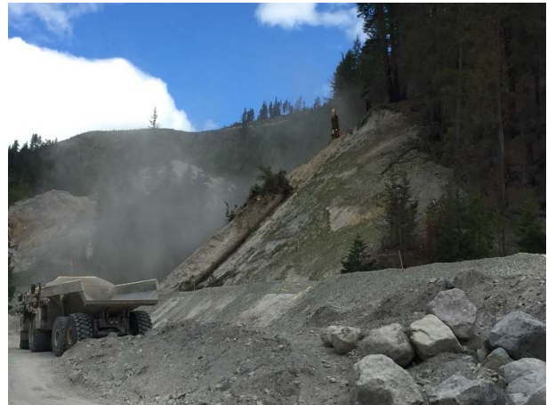
Photo 12 – Removing trees at the top of the cut slope above the penstock alignment on the left bank of Truckwash Creek (May 12, 2016).
