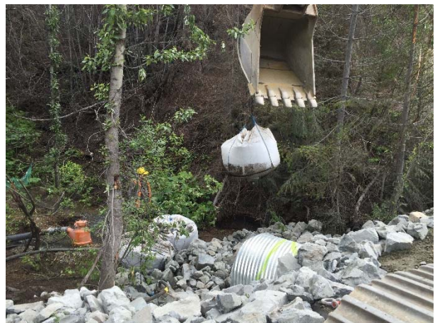
Photo 4– CE removing sand bags causing initial flush during commissioning of the new ASTR-04 culvert (May 20, 2016).
