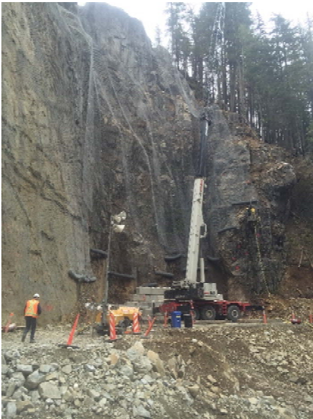
Photo 19 – Rock scaling and consolidation work above the future box canal location (May 18, 2016).
