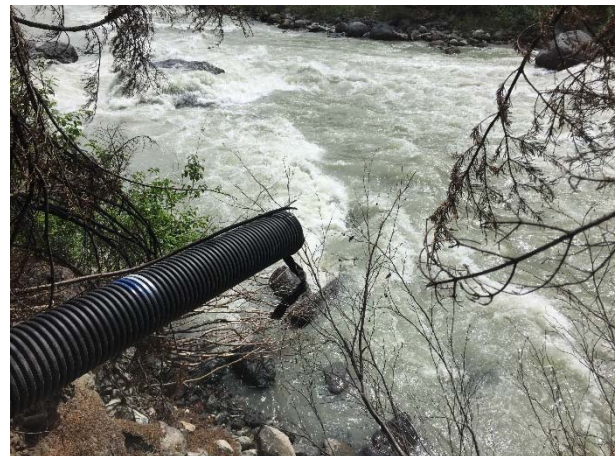
Photo 16 – Discharge to the Lillooet River from the water treatment system (May 15, 2016).
