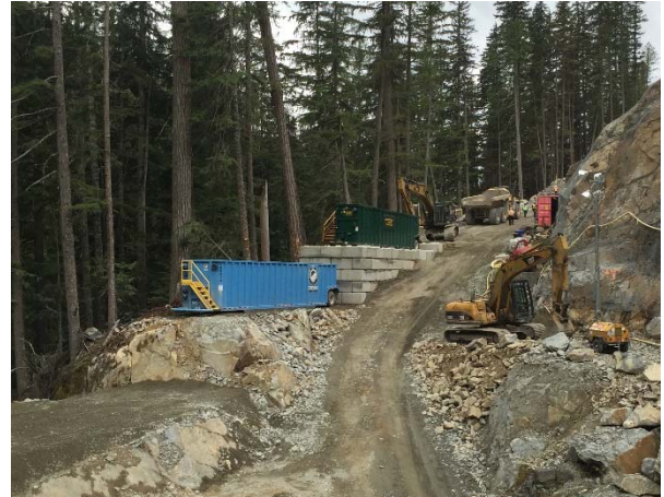
Photo 18 – Installation of the water treatment system along the edge of the BDRHEF intake access road (May 18, 2016).
