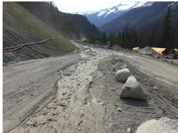
Photo 10 – Erosion and overland flow resulting from a power failure that caused the water treatment system to overflow and contribute elevated pH and turbid water to ASTR-03. The incident was reported as EIR#22 (May 15, 2016).
