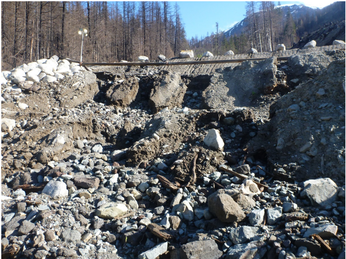
4. Another view of the erosion on site.
