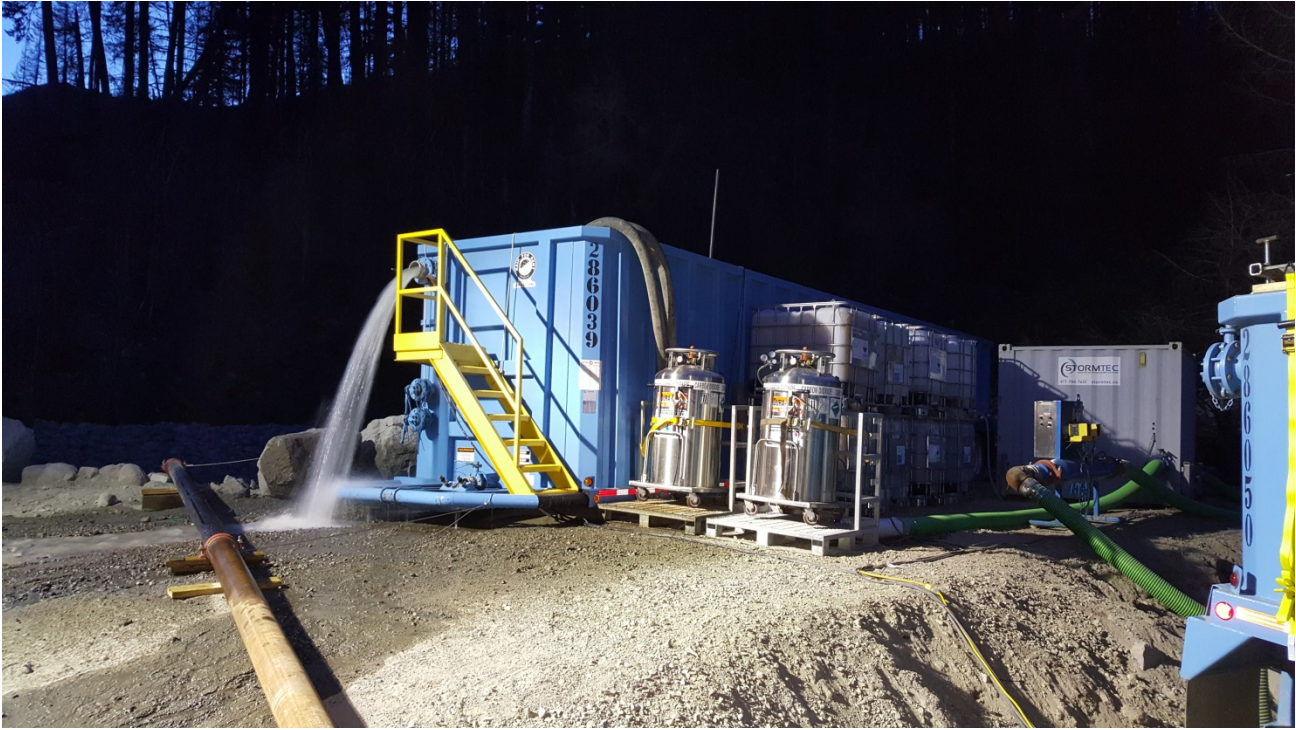
2. Water treatment tank overflowing
