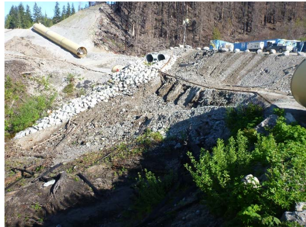
Photo 8 – Location of new active water treatment system and slope erosion resulting from a hose anchor failure reported as EIR#20 (May 5, 2016).
