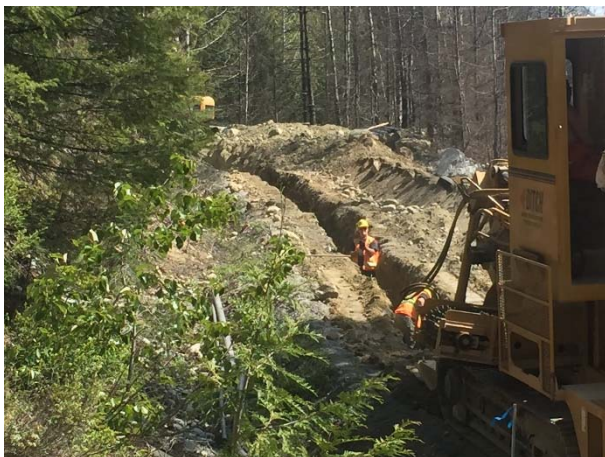
Photo 11 – Trenching for conduit installation in the BDRHEF intake access road outside of the UWR 500m buffer (April 29, 2016).
