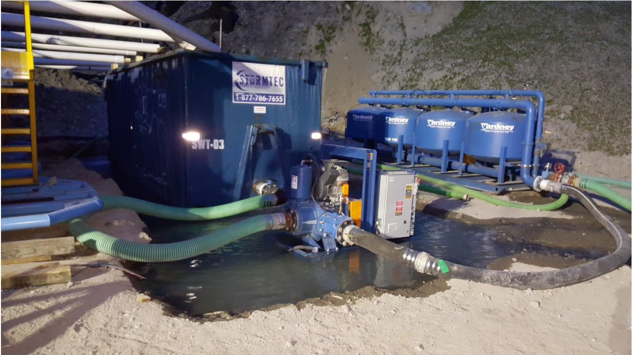
1. Flooded area near the sand filters
