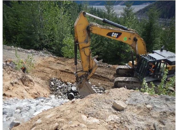
Photo 2 – Re-installation of the Pebble Creek Main road culvert performed under IEM supervision (April 24, 2016).
