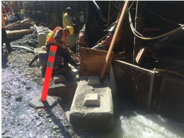
Photo 3 – CE crew attempting to isolate the clean water sump during the concrete arch foundation wall mudslab pour (May 02, 2016).
