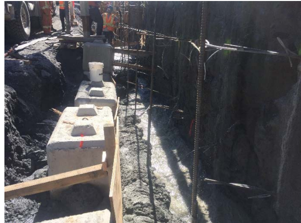
Photo 4 – Concrete arch foundation wall mudslab pour was abandoned as the seepage water could not be controlled (May 02, 2016).
