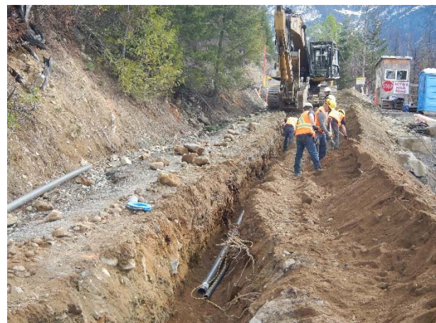
Photo 13 – Conduit installation in the BDRHEF intake access road outside of the UWR 500m buffer (April 22, 2016).
