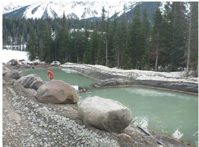
Photo 6 – Pond 6 and 7 of ULR upstream tunnel portal treatment system (April 17, 2016).
