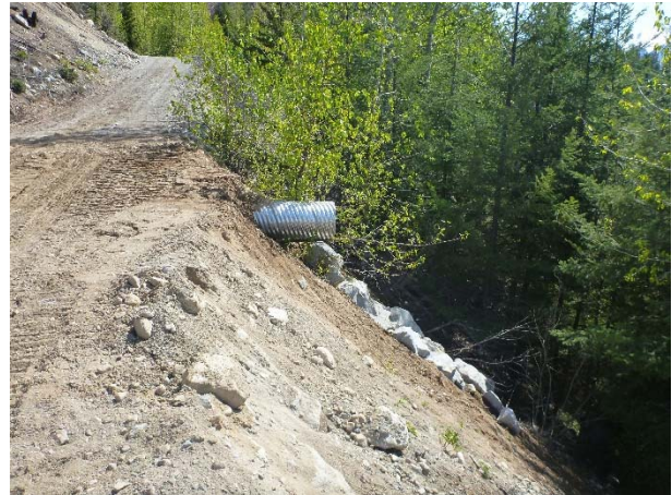
Photo 2 – Perched culvert with inadequate outlet armoring (April 18, 2016).
