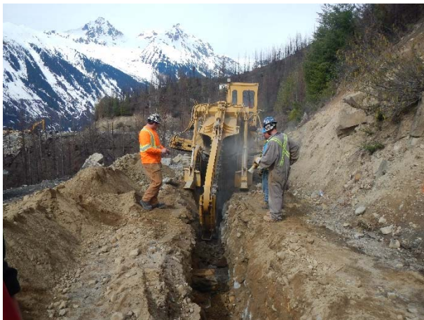
Photo 12 – Trenching for conduit installation in the BDRHEF intake access road outside of the UWR 500m buffer (April 22, 2016).
