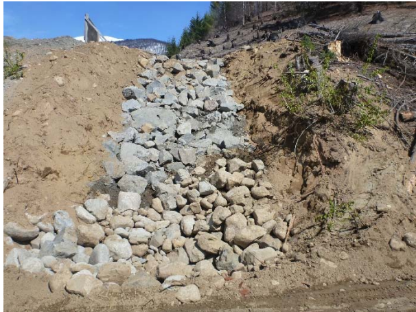
Photo 1 – Over-sized riprap on slope above culvert inlet (April 18, 2016).
