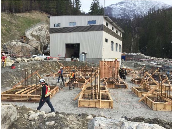
Photo 13 – Current conditions at the BDRHEF tunnel portal, powerhouse, and switch yard (April 04, 2016).
