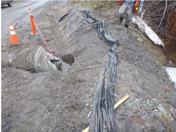
Photo 1 – Damaged culvert at KM43 of the Lillooet River FSR (April 7, 2016).
