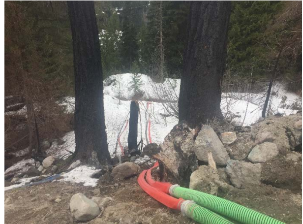
Photo 10 – Outlet hoses from the new water treatment system discharge directly to ASTR-03 (April 2, 2016).
