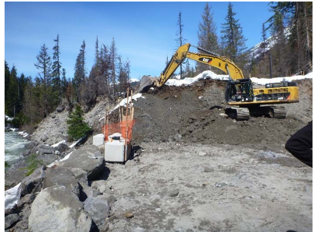
Photo 12 – Excavation of the top of the natural earth berm separating the ULRHEF tailrace from the Lillooet River (April 8, 2016).
