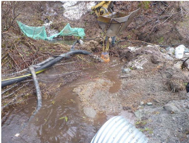
Photo 3 – Turbid water associated with the placement of diversion pump at KM43 (April 7, 2016).
