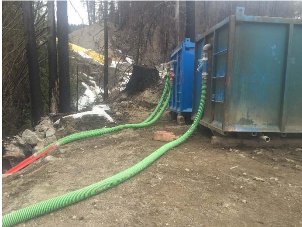
Photo 9 – ULRHEF downstream tunnel treatment system, installed on April 2, 2016.
