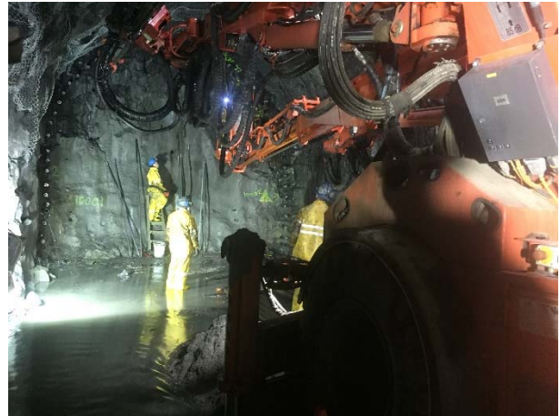
Photo 6 – Canopy tube installation; a component of the umbrella support system being installed within the ULRHEF upstream tunnel (March 23, 2016).
