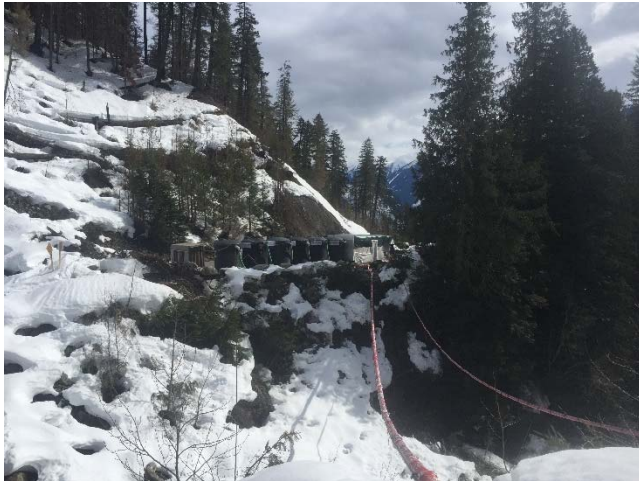
Photo 7 – Active water treatment system at the downstream tunnel infiltration ponds (March 22, 2016).
