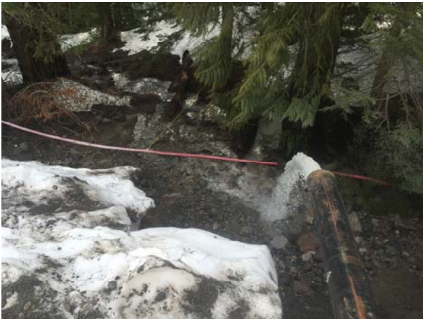
Photo 3 – Turbid discharge that is not able to be fully captured by the active water treatment system at Truckwash Creek is being directed offsite, over the edge of a cliff, and ultimately connects to the Lillooet River. The discharge presents an ESC risk to downstream areas and exceeds BCWQGs for pH and turbidity. Please install appropriate ESC and pH mitigation measures until a large capacity water treatment system is installed. (March 23, 2016)
