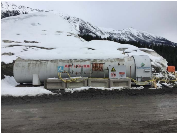
Photo 3 – Installation of the bulk CO 2 system to support the water treatment system at the ULRHEF intake was completed and active as of March 19, 2016.
