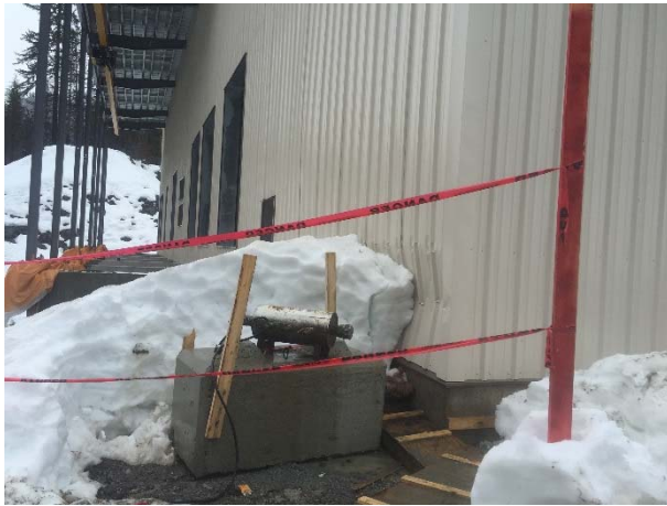
Photo 11 – Minor snow damage resulting from snow sliding off the roof of the ULRHEF powerhouse (March 23, 2016).
