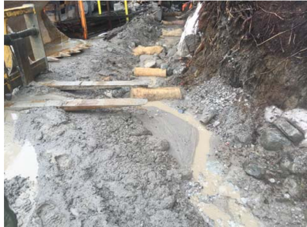
Photo 2 – Measures installed by CE to treat turbid water in the ditch line are not functioning as intended. Please ensure all water from this ditch line is directed to the water treatment system until material required to fix the ditch line is available. (March 23, 2016)
