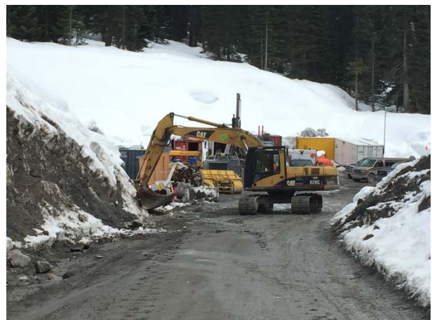
Photo 2 – Snow removal and ditch maintenance near KM49 of the Lillooet River FSR (March 19, 2016).
