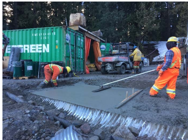
Photo 10 – CE installed a concrete pad in front of culvert that is intended to intercept road and work site runoff and direct it to the active water treatment system (ULR#43; March 25, 2016).
