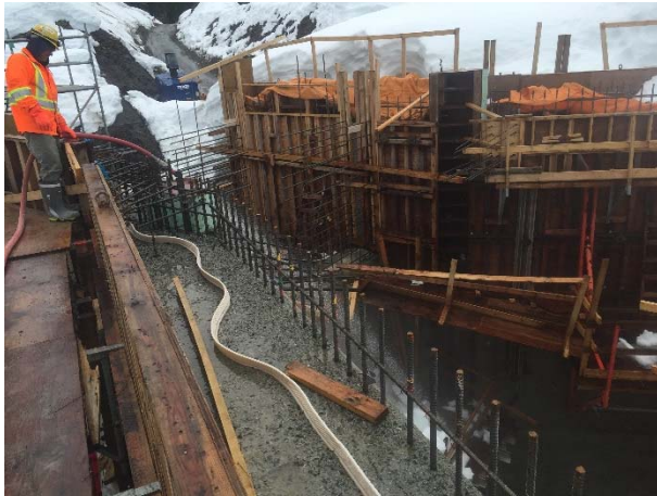
Photo 5 – Spraying hot water to melt snow at the ULRHEF intake structure (March 23, 2016).
