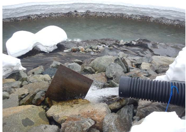
Photo 4 – Discharge from ULRHEF sediment basins to Lillooet River during canopy tube installation (drilling) in the tunnel (March 8, 2016).
