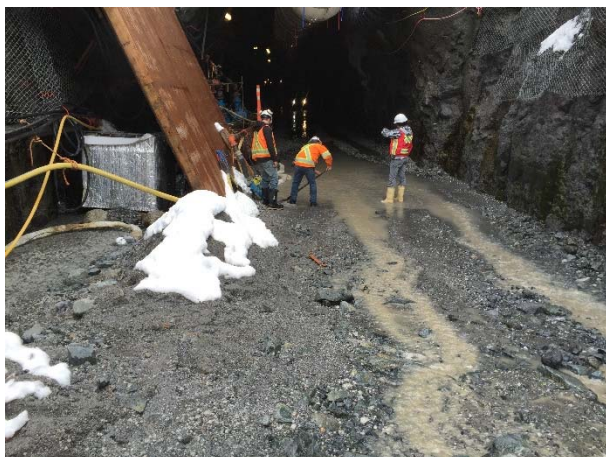
Photo 5 – Working to isolate turbid road runoff from the clean water sump. The turbid runoff resulted in a temporary exceedance of BCWQGs in the Lillooet River (March 11, 2016).
