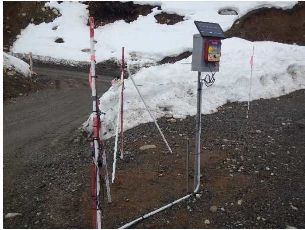
Photo 1 – Electric fence on Pad 1 (March 8, 2016).
