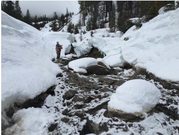
Photo 9 – Failure of the outside wall of the sediment pond caused by a small snow and debris slide into the pond (March 12, 2016).
