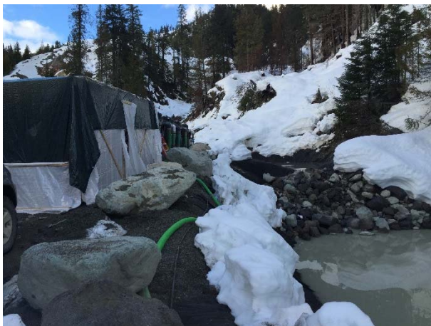
Photo 7 – Active water treatment system at the downstream tunnel infiltration ponds (March 7, 2016).
