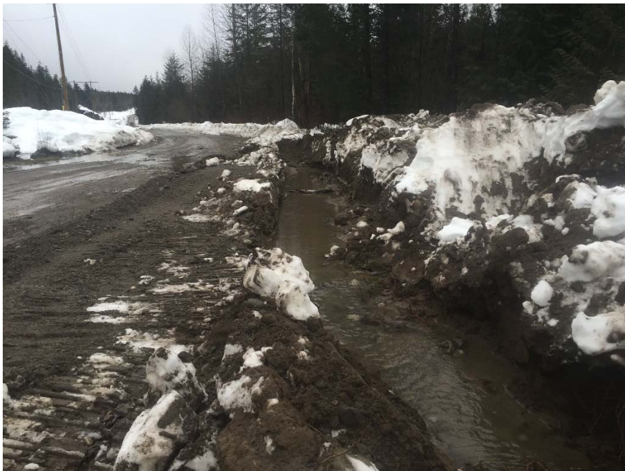
Photo 2. Water crossing the road is conveyed downstream in a new ditch line excavated parallel to the FSR. February 17, 2016
