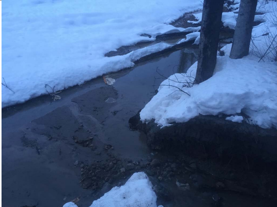
Photo 5 – Looking upstream at the confluence of the new channel and Lillooet River side channel. February 17, 2016
