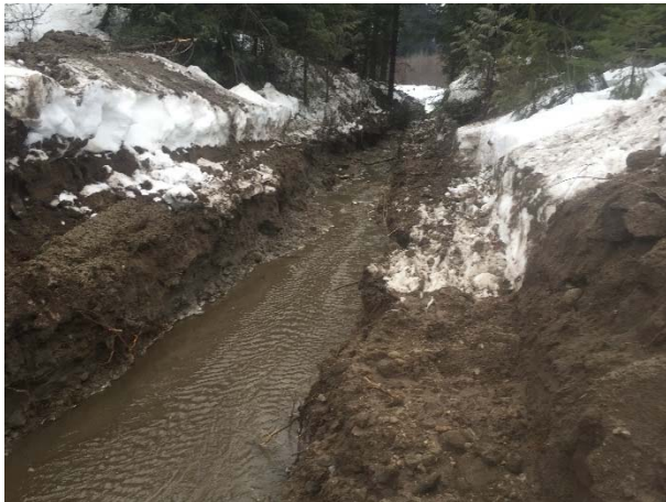
Photo 3 – Ditch excavated by CE at KM21 of the Lillooet River FSR (February 15, 2016).
