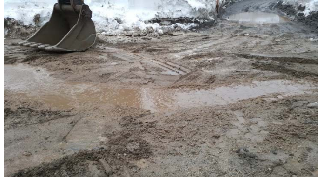
Photo 2 – CE installed a cross ditch to address runoff issues at KM48 on the Lillooet River FSR. Road runoff was directed to a vegetated area and away from the cuthroat trout stream (February 19, 2016).
