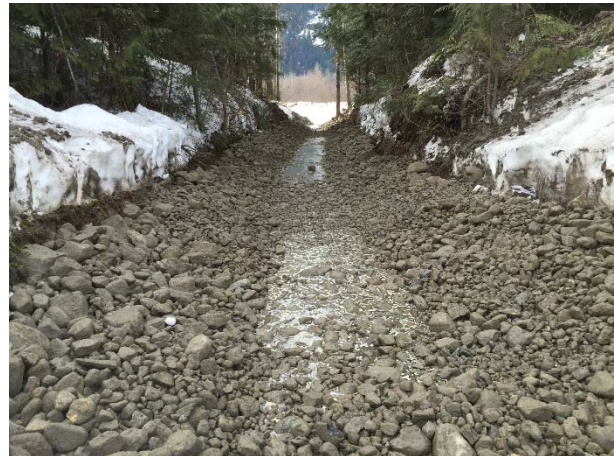
Photo 4 – Repairs completed under IEM supervision to stabilize the ditch at KM21 of the Lillooet River FSR (February 25, 2016).
