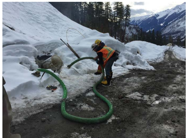
Photo 12 – Repairing a hole in a hose in the water treatment system hose (February 26, 2016).
