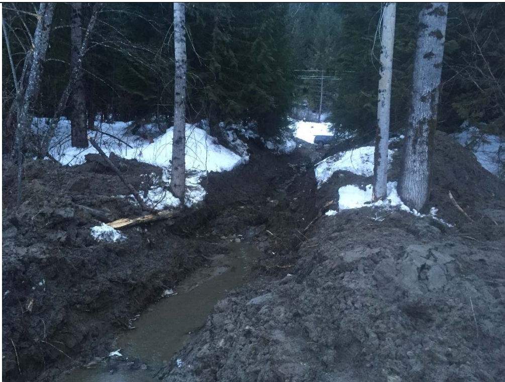
Photo 4. Looking back toward the Lillooet River FSR from the terminus of the newly excavated channel. February 17, 2016
