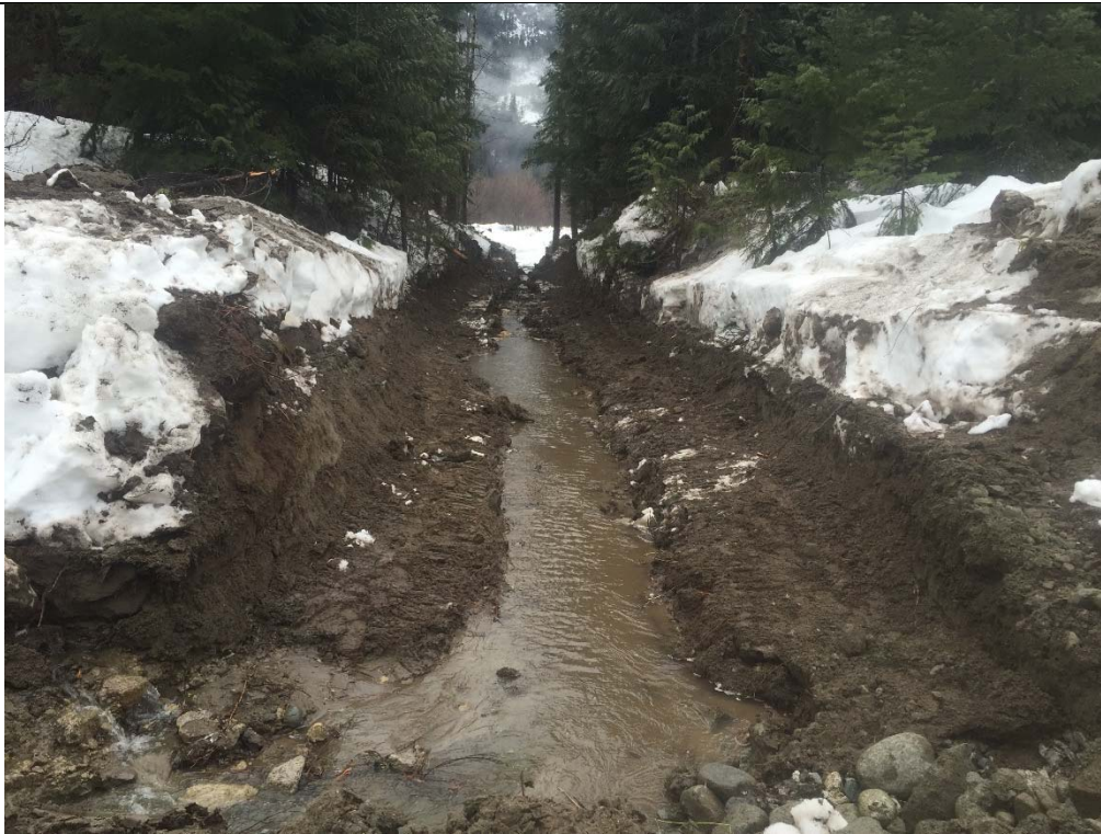
Photo 3. Water flowing along the road side ditch turns a corner here and heads towards the Lillooet River in this newly excavated channel. This channel is composed of highly erodible material that requires armouring to be protected from erosion. February 17, 2016
