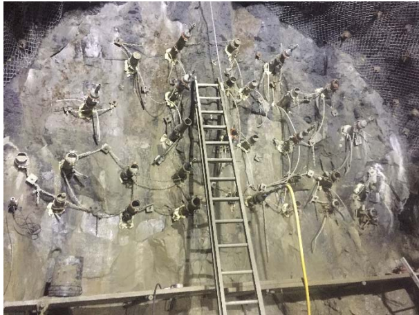
Photo 5 – The face of the ULRHEF upstream tunnel during tunnel cover grouting (February 24, 2016).
