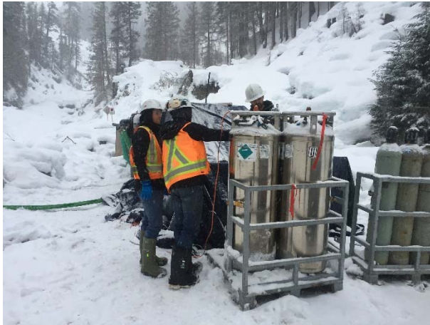
Photo 5 – Installation of active water treatment system at the downstream tunnel infiltration ponds (February 3, 2016).
