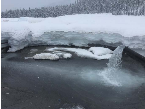
Photo 2 – The first cell of the ULRHEF sediment basins during tunnel grouting (February 3, 2015).
