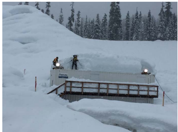
Photo 6 – Snow removal off buildings at the ULRHEF intake (January 30, 2016).
