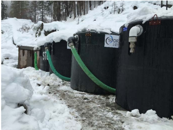
Photo 15 – Settling tank portion of the water treatment system (January 27, 2016).
