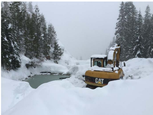
Photo 13 – Excavator clearing a pad for installation of the Stormtec water treatment system (January 18, 2016).
