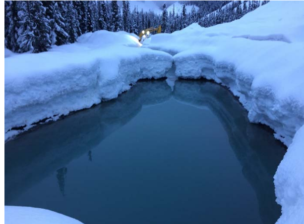
Photo 10 – The IEM conducted sampling for pH in the last cell (Pond 7) of the ULRHEF sediment basins during tunnel grouting (January 26, 2016).
