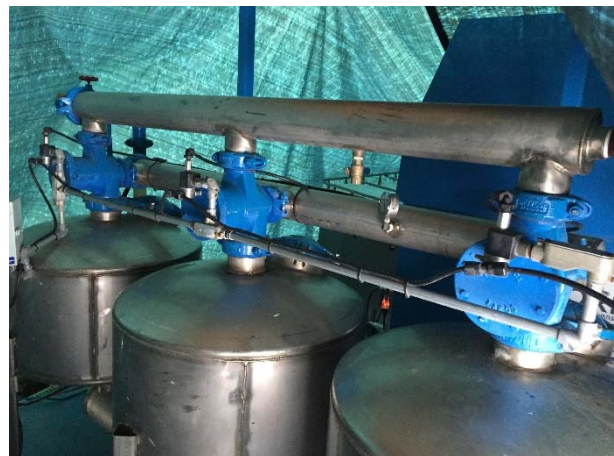
Photo 14 – The sand filter stage of the water treatment system (January 29, 2016).
