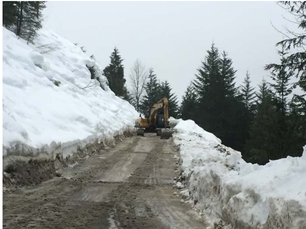
Photo 7 – Cross ditching at KM0.75 of the camp access road (January 27, 2016).
