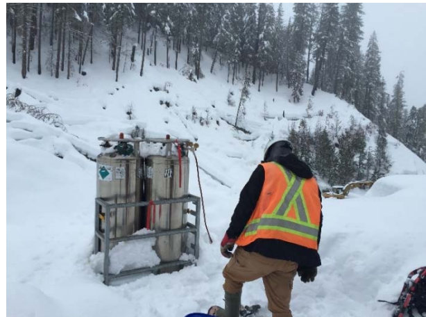
Photo 12 – CO 2 diffuser installed to treat elevated pH in the oil/water separator (January 18, 2016).
