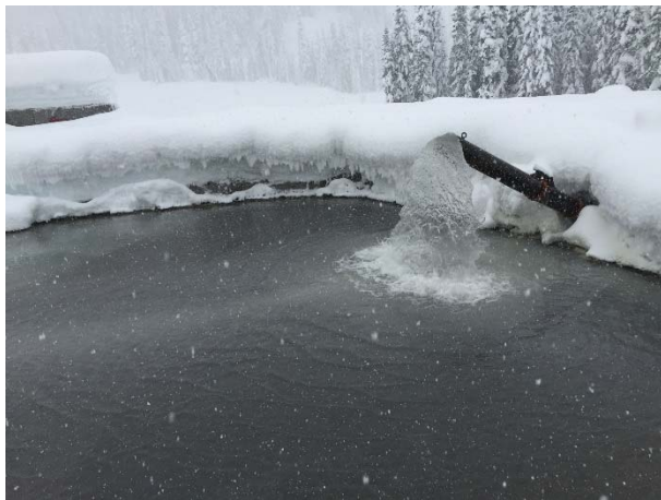
Photo 5 – Water being directed to the first cell of the of the ULRHEF sediment basins during tunnel grouting (January 12, 2016).
