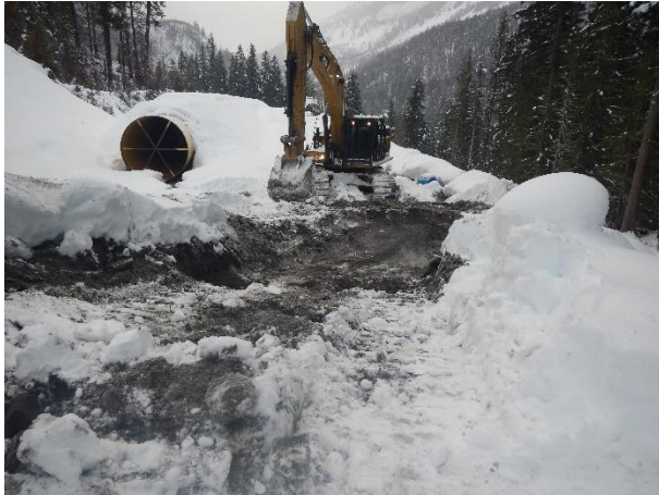
Photo 4 – Repairing the outlet of the ULRHEF downstream tunnel infiltration ponds at Truckwash creek (December 15, 2015).
