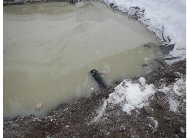
Photo 5 – Plugged outlet pipe at the ULRHEF downstream tunnel infiltration ponds (December 15, 2015).
