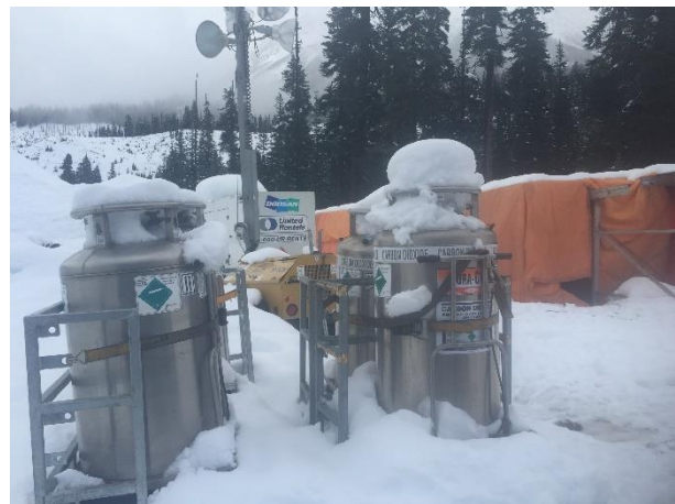
Photo 2 – Active water treatment system with CO 2 tanks at ULRHEF intake sediment basins (December 9, 2015).
