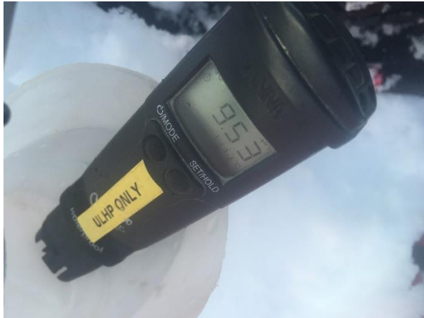
Photo 3 – The IEM conducting sampling for pH in the first sediment basin pond during grout injection works (December 9, 2015).
