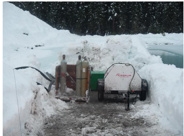
Photo 6 - Secondary Sumas water treatment system at Pond 5 of ULRHEF intake basins (December 4, 2015).
