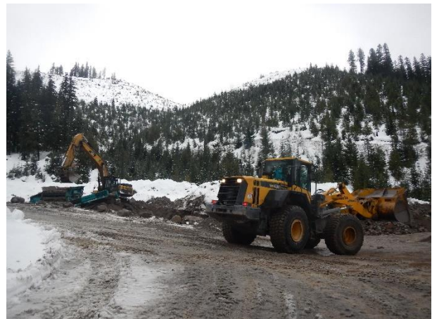
Photo 2 – Screening material at the spoil pile located at KM45 of the Lillooet River FSR. Screened material was stockpiled and used to sand the FSR (December 4, 2015).
