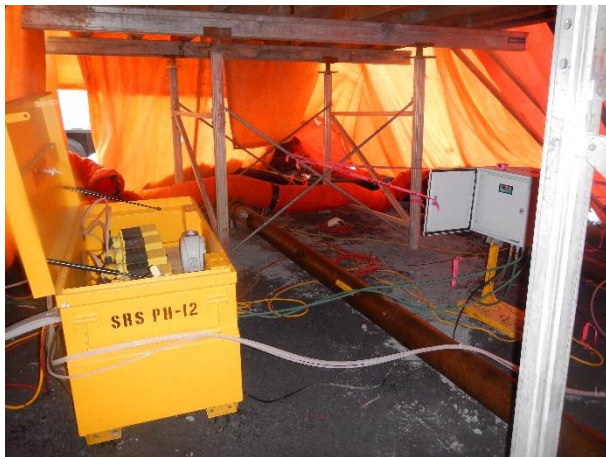
Photo 5 – Primary Sumas water treatment system near Pond 2 of ULRHEF intake basins (December 4, 2015).
