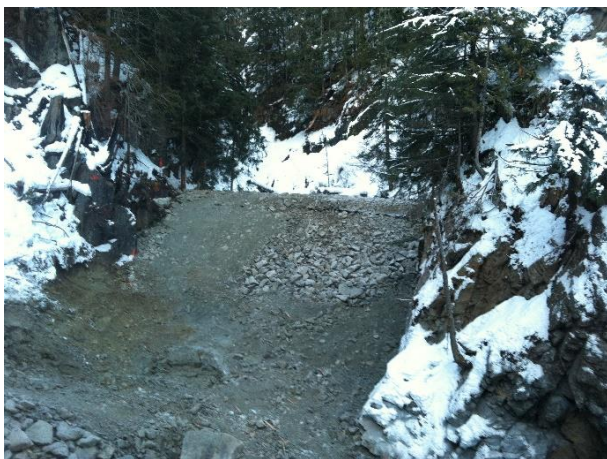
Photo 11 – Upstream cofferdam at BDRHEF Intake (November 30, 2015).
