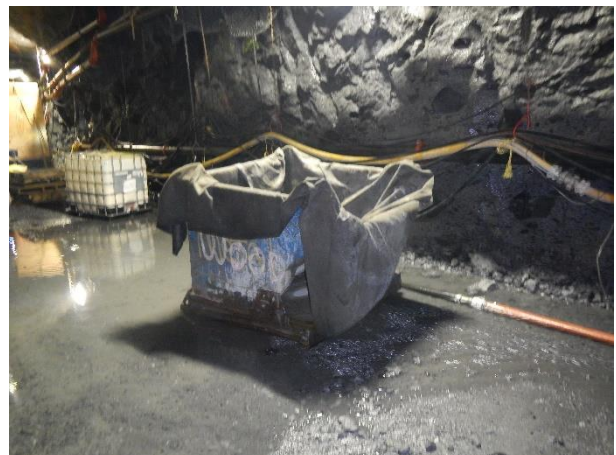
Photo 8 – Geotextile-lined bins used in the tunnel to dispose of excess grout (December 5, 2015).
