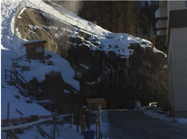
Photo 28 – BDRHEF tunnel portal closed during this reporting period due to blasting restrictions (November 27, 2015).
