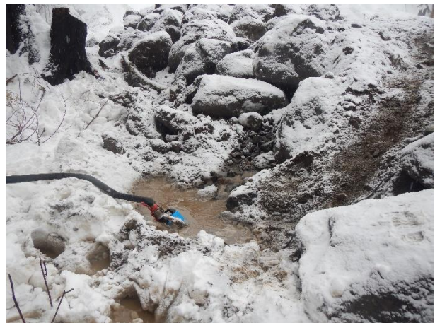
Photo 8 – Seepage noticed at downstream end of reconstructed channel indicative of sub-surface flows (November 23, 2015).
