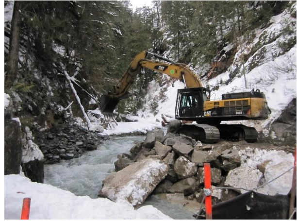
Photo 14 – Excavator equipped with biodegradable hydraulic oil removing upstream end of diversion channel (November 22, 2015).
