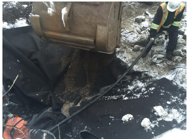
Photo 6 – Placement of impermeable geotextile membrane and backfill of the existing bypass sump while continuing to bypass the majority of flows (November 23, 2015).
