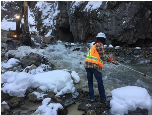
Photo 26 – Water quality sampling downstream of the diversion tunnel during downstream cofferdam construction (November 28, 2015).
