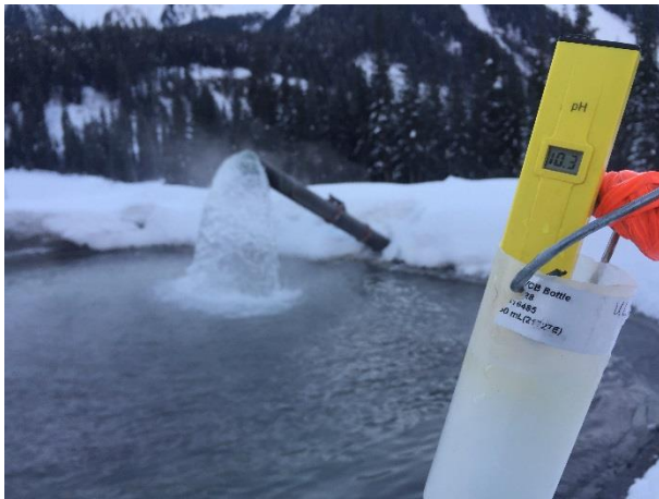
Photo 1 – Alkaline water pumped to ULRHEF intake sediment basins during grout injection (November 28, 2015).
