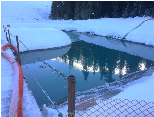
Photo 3 – Orange hose (foreground) conveying water to CO 2 treatment system and hose (background) pumping water through diffuser pipe and back to ponds (November 28, 2015).
