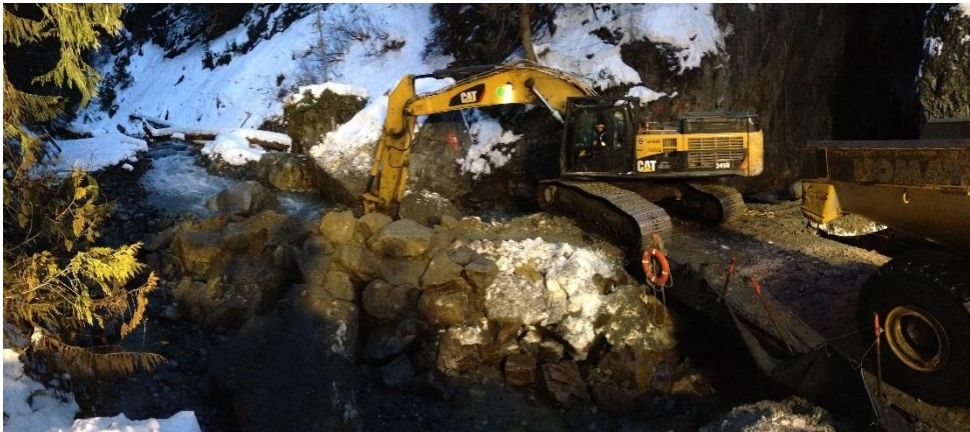
Photo 15 – Upstream cofferdam with excavator removing plug releasing majority of creek flow to diversion tunnel (November 22, 2015).
