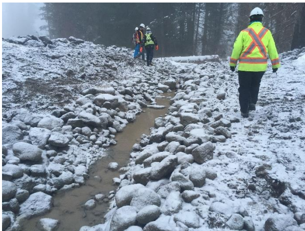
Photo 5 – Initial re-watering of ASTR-04 overdrain by bypass pump to permit working on the placement of an impermeable geotextile membrane and backfilling to grade (November 23, 2015).
