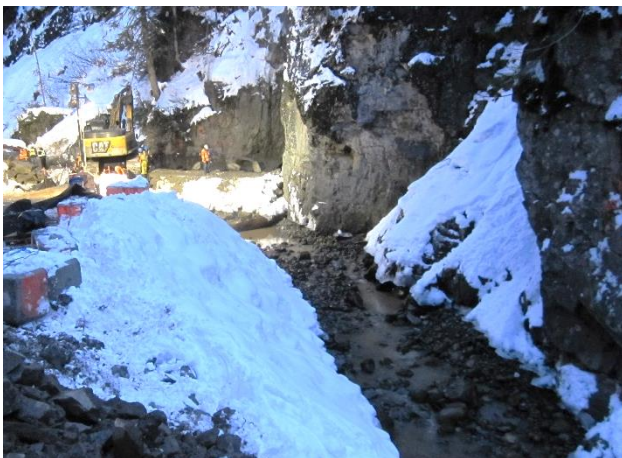
Photo 16 – View looking upstream at dewatered creek channel following plug removal and diversion of flow (November 22, 2015).
