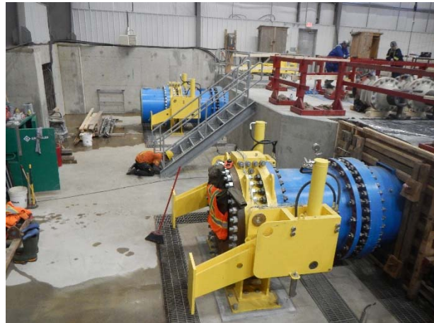
Photo 19 – View inside the BDRHEF powerhouse (November 17, 2015).
