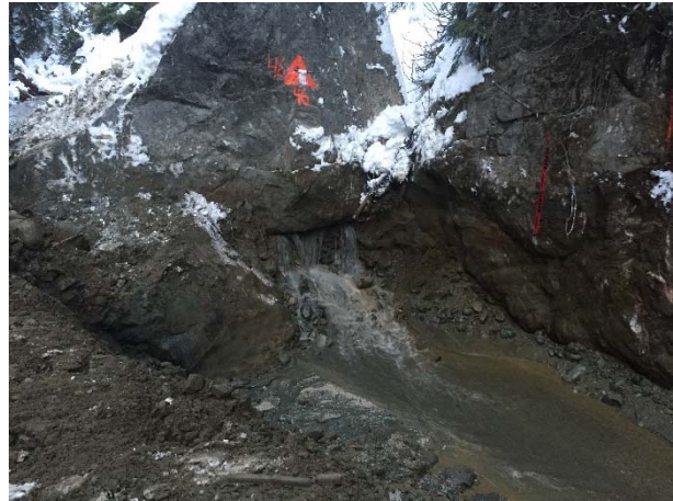
Photo 14 – Large boulder restricting flow to BDRHEF intake diversion tunnel (November 21, 2015).
