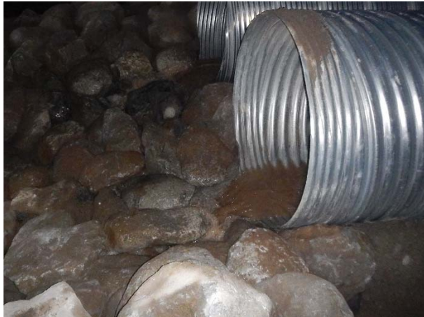
Photo 18 – Turbid flows through over-drain culverts following construction of ASTR03 over-drain berm (November 8, 2015).
