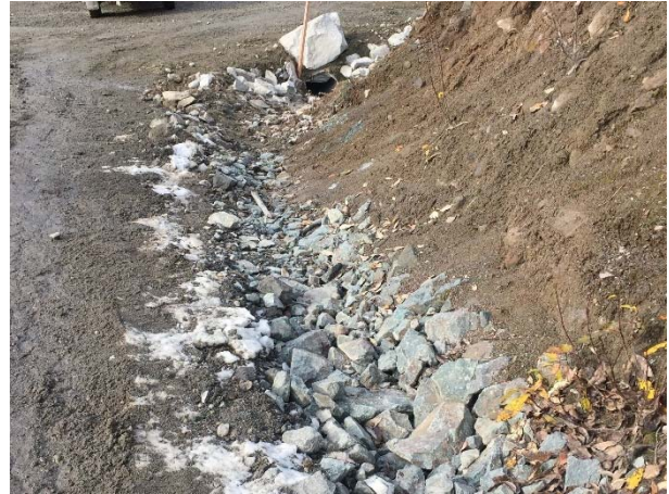
Photo 2 – Ditching completed and culvert installed at KM 45 on the Lillooet River FSR (November 11, 2015).
