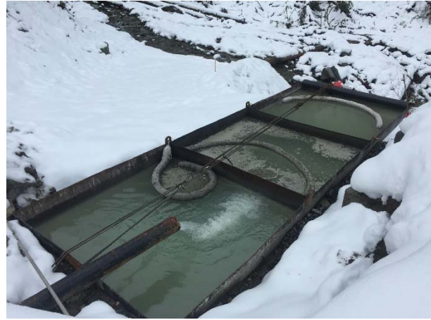
Photo 13 – Oil-water separator at ULRHEF downstream portal (November 14, 2015).
