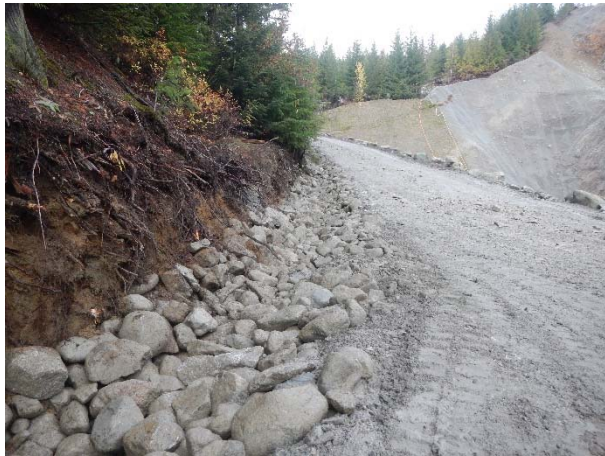
Photo 14 – Ditch maintenance and rock lining completed on downstream portal access road (November 8, 2015).
