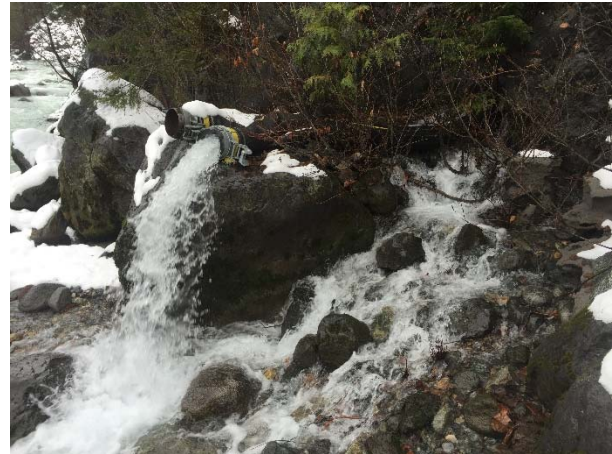
Photo 29 – Dewatering seepage water from the ULRHEF powerhouse sump to the Lillooet River (November 14, 2015).
