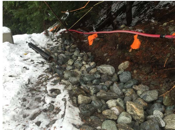
Photo 15 – Ditch maintenance and rock lining completed on downstream portal access road (November 14, 2015).
