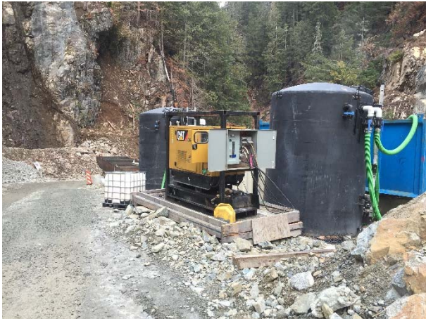
Photo 32 – Active water treatment system at BDRHEF intake (November 10, 2015).
