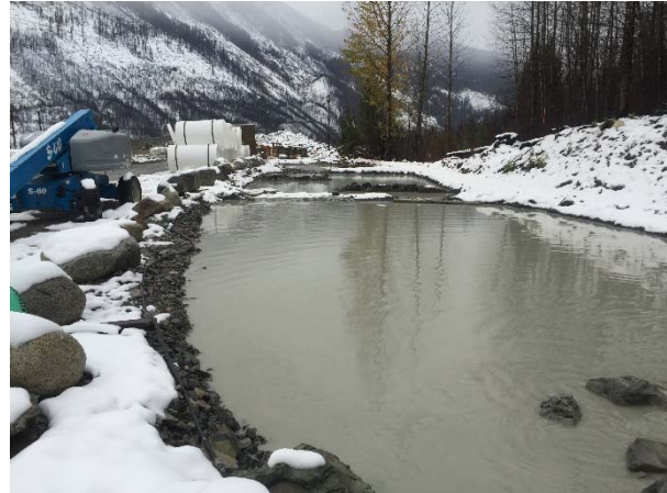
Photo 36 – BDRHEF tunnel portal settling ponds (November 14, 2015).
