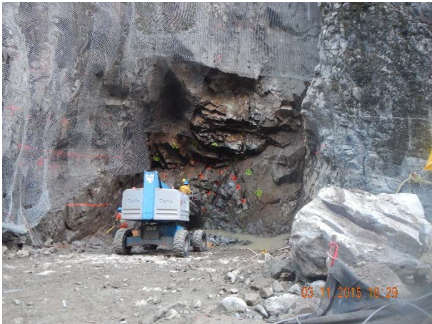
Photo 21 – Loading drilled holes with explosives prior to the diversion tunnel blast (November 3, 2015).
