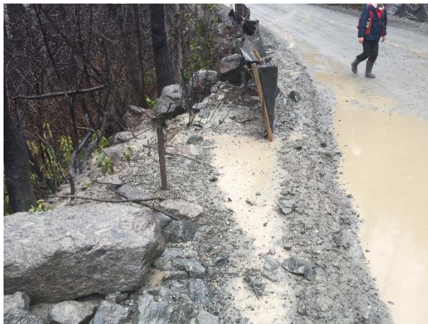
Photo 16 – Turbid road runoff entering ASTR04 (November 6, 2015)
