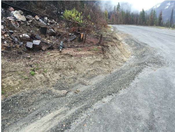
Photo 1 – Ditch work completed between KM43.5 – KM44 of the Lillooet River FSR (November 1, 2015).
