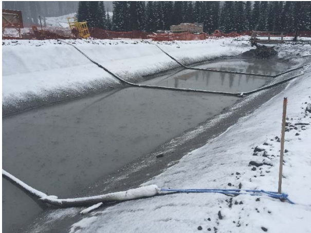
Photo 6 – Oil/water separator section of the ULRHEF intake sediment basins (November 6, 2015).
