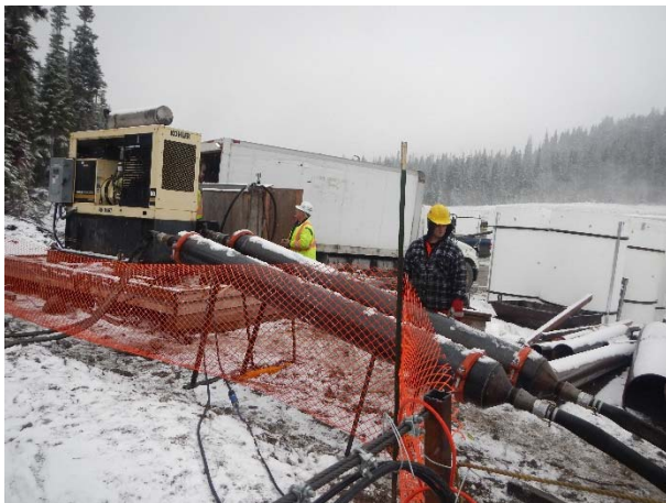
Photo 8 – Installing a more robust flocculant injection system and cell #2 of the ULRHEF intake sediment basins (November 6, 2015).
