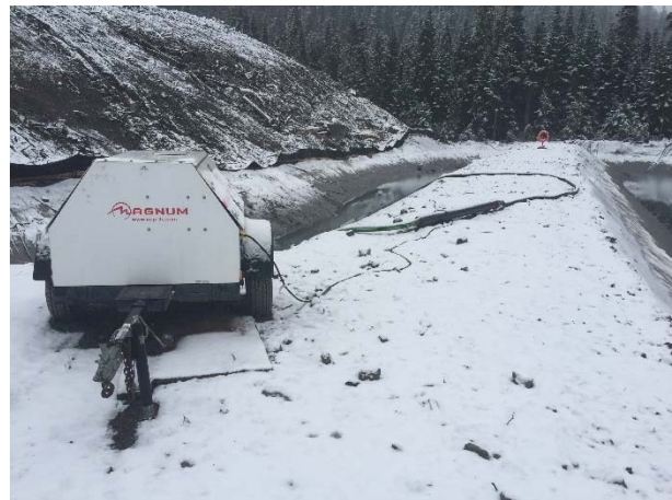
Photo 9 – Secondary flocculant injection system installed at ULRHEF intake sediment basins was functioning throughout the reporting period (November 6, 2015).
