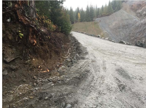
Photo 11 – CE performed maintenance of the ditch along the ULRHEF downstream portal access road (November 6, 2015).
