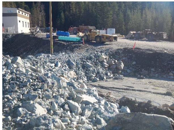
Photo 26 – Blast rock placed to prevent seepage from the 4 th cell of the BDRHEF tunnel portal settling ponds from impacting the haul path. (November 5, 2015).
