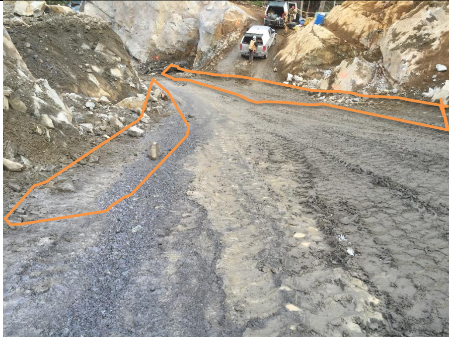
BDR#27. Ditches outlined in the work plan have not been installed and sediment/sediment laden water are flowing over the running surface along the length of the ramp
