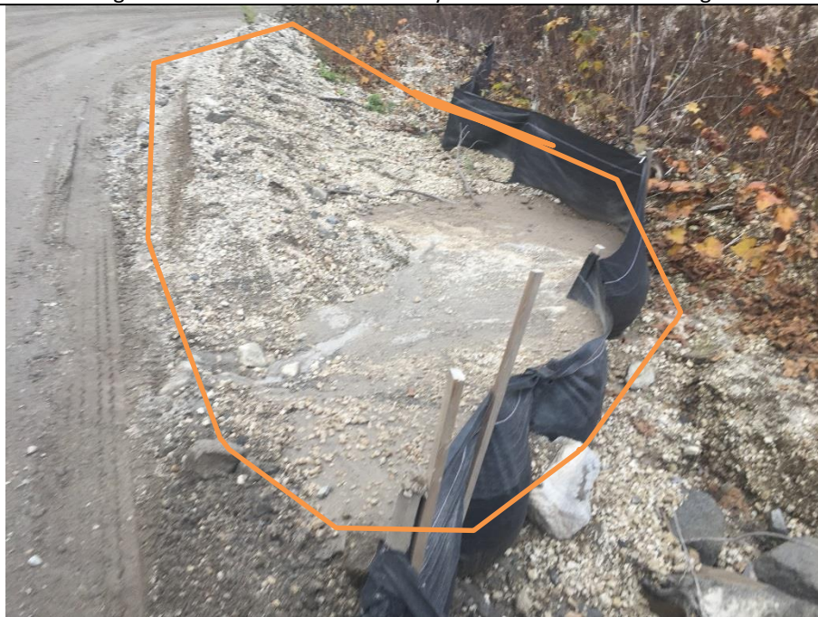
ULR#32. The silt fence on the upstream side of the second WBC is 95% infilled with sediment and has previously failed (KM48 of the Lillooet River FSR).
