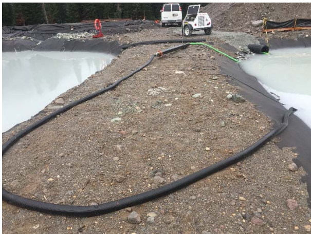
Photo 11 – Flocculant injection system installed at ULRHEF intake sediment basins (October 28, 2015).
