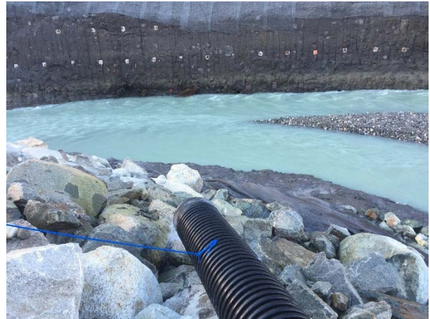
Photo 10 – ULRHEF intake sediment basin outlet pipe at Lillooet River (October 26, 2015).
