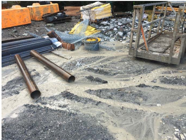
Photo 15 – Turbid runoff fanning out in laydown area at bottom of downstream portal access road (October 31, 2015).
