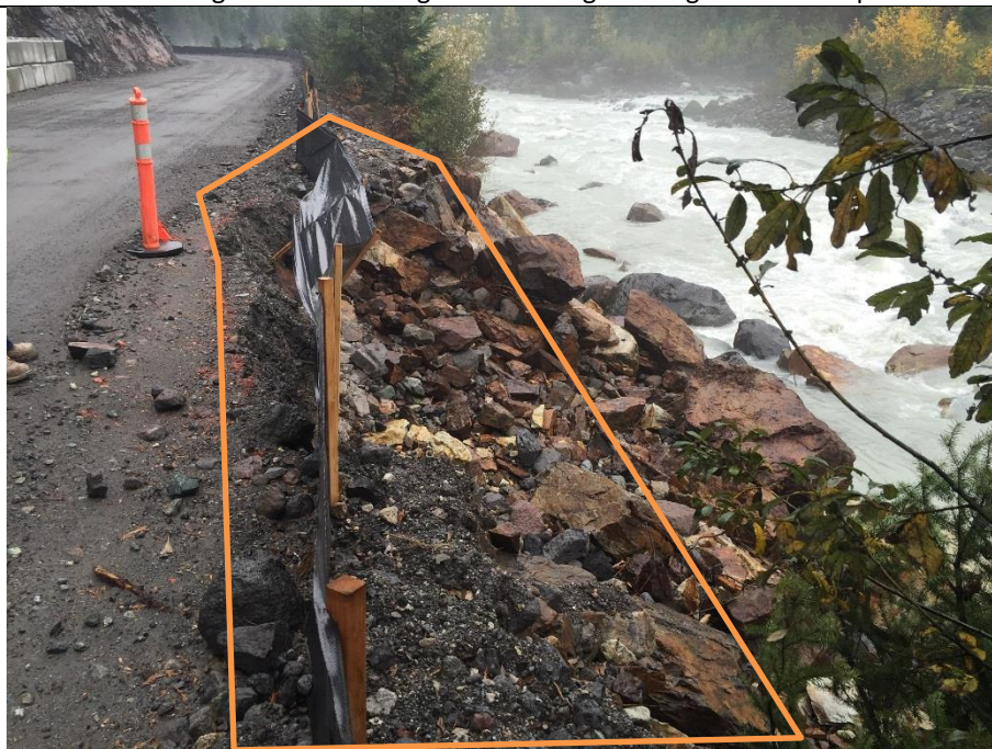
ULR#28. The road edge eroded significantly during scaling activities and during the last major rain event and requires bank stabilization (above the HWM), ditch installation/maintenance, and silt fence repair.
