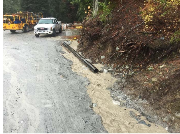
Photo 14 – Turbid runoff in ditch on ULRHEF downstream portal access road (October 31, 2015).
