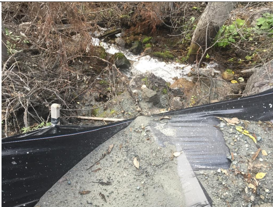
ULR#30. The silt fence on the downstream side of the WBC/road at ASTRO4 has failed. Runoff from the surface of the haul road is not conveyed in a ditch. As a result flows concentrate in this location, which led to the silt fence failure.
