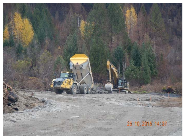
Photo 4 – Construction of PAG stockpile area at KM 41.75 on the Lillooet River FSR (October 25, 2015).
