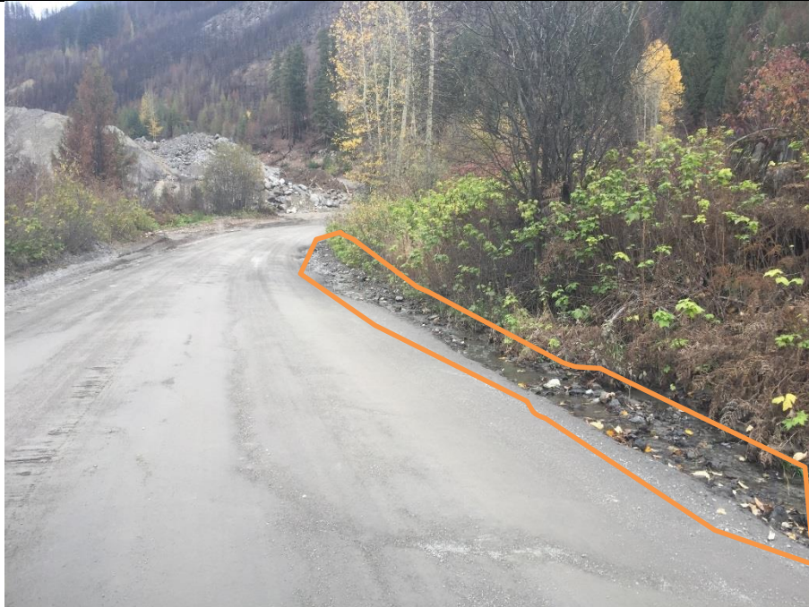
ULR#29. Water in the ditch line is eroding the road edge
