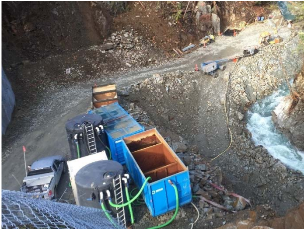
Photo 27 – Active water treatment system at BDRHEF intake (October 29, 2015).
