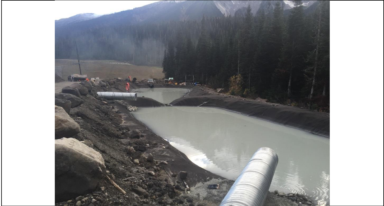
ULR#34. The flocculant and pH treatment components of the water treatment ponds are not currently installed
