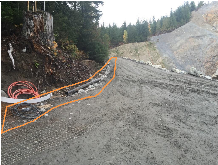
ULR#31. Ditches are not collecting and transporting road runoff as intended due to the road grading along the lower ULRHEF tunnel portal access road and infilling of the ditch line. Surface runoff is not conveyed in ditch lines and discharges sediment laden water directly to Truckwash Creek during rain events.
