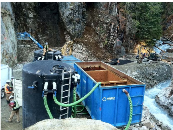
Photo 17 – Installation of the Sumas water treatment system in preparation for tunneling activities (October 23, 2015)
