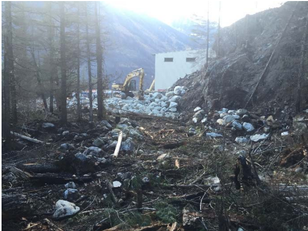
Photo 21 – Armouring of the upstream end of the BDRHEF powerhouse flood protection berm (October 9, 2015).
