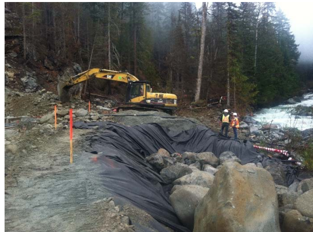
Photo 20 – Construction fo the toe of the BDRHEF powerhouse flood protection berm (October 18, 2015).
