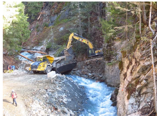
Photo 18 – Excavation in isolation of flowing water at the upstream diversion tunnel portal face (October 24, 2015)
