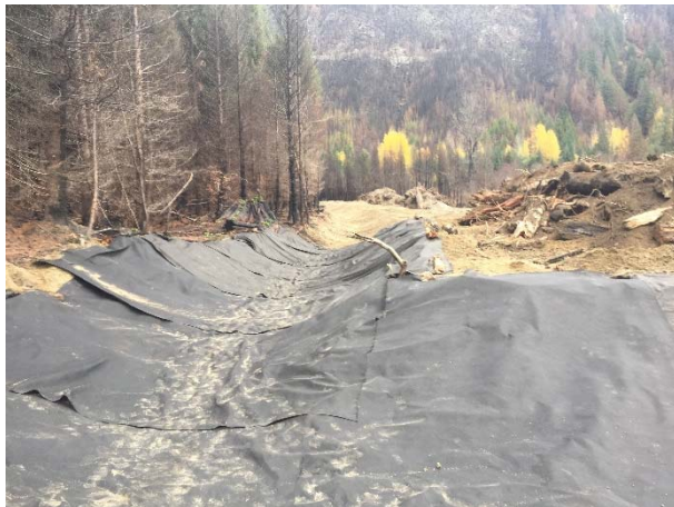
Photo 1 – Ditching and drainage armouring around the permanent PAG rock storage area. (October 22, 2015).
