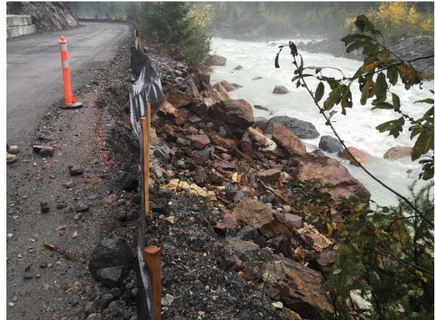
Photo 4 – Road stabilization works required at KM 41 on the Lillooet River FSR (October 8, 2015).
