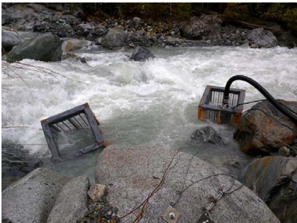
Photo 21 – Fish exclusion boxes re-installed on pump intakes in Boulder Creek (October 9, 2015).
