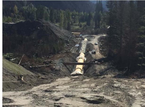
Photo 7 – Overview of active penstock work area; including welding and backfill placement (September 29, 2015).
