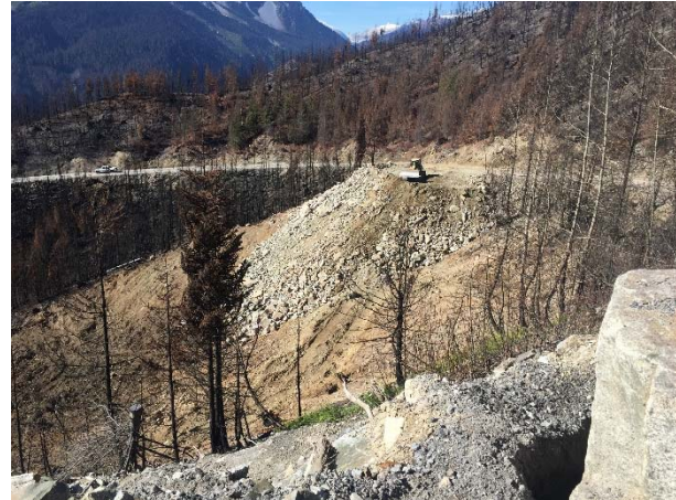
Photo 11 – Spoil area used to place blast rock generated from the intake access ramp excavation. (September 29, 2015).
