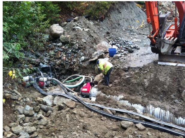
Photo 15 – Pumps and hoses installed to dry work area during the 272a culvert removal. Once the culvert was dry it was assessed for CTF presence (October 2, 2015)
