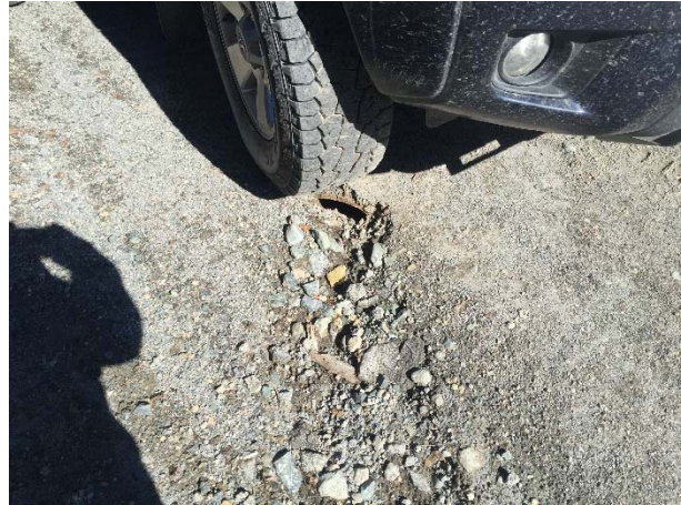
Photo 4 – Culvert outlet from the ULRHEF downstream tunnel portal infiltration ponds has been buried and requires repair. (September 29, 2015).
