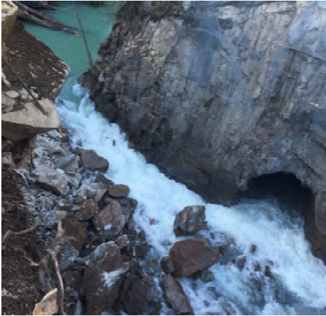
Photo 10 – Material lost during blasting for the excavation of the access ramp at BDRHEF intake. Water quality remained visually unaffected immediately after the blast. (September 27, 2015).
