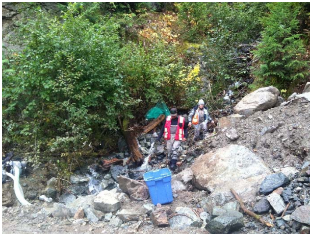
Photo 14 – Installing CTF isolation netting and conducting CTF salvage prior to starting the stream 272a culvert removal works in Segment 11. (October 2, 2015).
