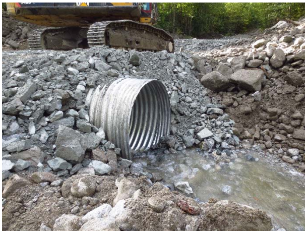
Photo 3 – Culvert replaced at at 31 KM on the Lillooet River FSR following washout (September 21, 2015).
