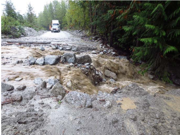
Photo 1 – Washout at 31KM on the Lillooet River FSR (September 20, 2015).
