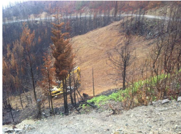
Photo 21 – Grubbing and stripping for spoil area at KM 3 on the BDRHEF intake access road (September 16, 2015).
