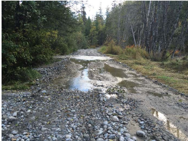
Photo 26 – Flooding on South Lillooet FSR due to beaver and flooding activity (September 25, 2015).
