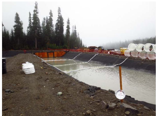
Photo 7 – ULRHEF intake sediment basins (September 18, 2015).
