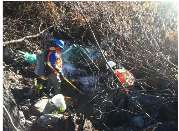
Photo 4 – Fish salvage conducted by Ecofish prior to installation of log box culvert (September 11, 2015).
