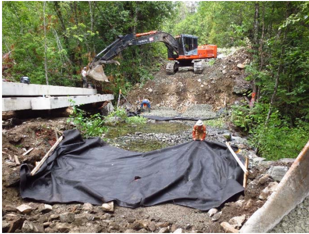
Photo 26 – Preparation for installation of precast footings and steel columns at MB53 (September 1, 2015).
