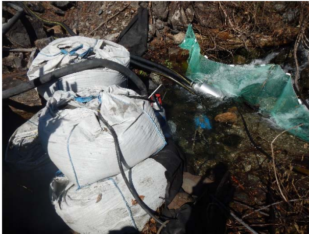
Photo 5 – Sandbag berm and pumps used to isolate box culvert work area from water (September 11, 2015).
