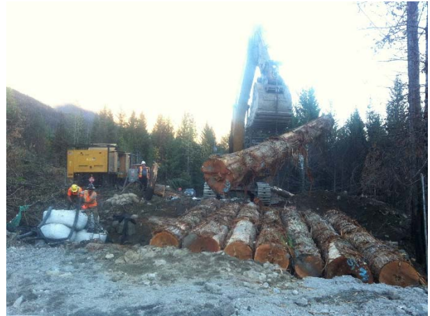
Photo 6 – Installation of the log box culvert on the magazine access road (September 12, 2015).
