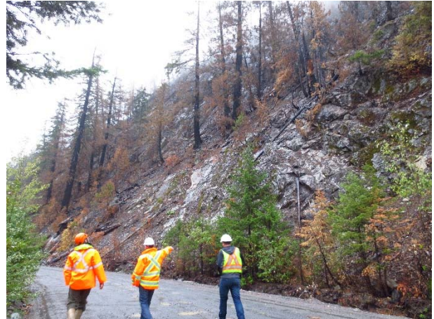
Photo 2 – Kick-off meeting held for scaling and danger tree removal works at KM 41 on the Lillooet River FSR (September 2, 2015).
