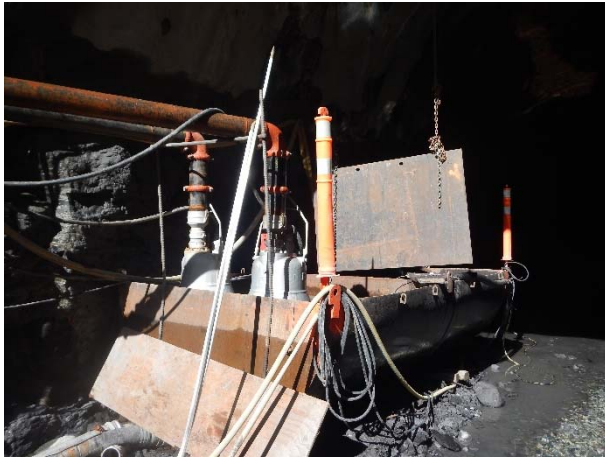
Photo 9 – Sump box and pumps installed at entrance to upstream tunnel portal (September 12, 2015).
