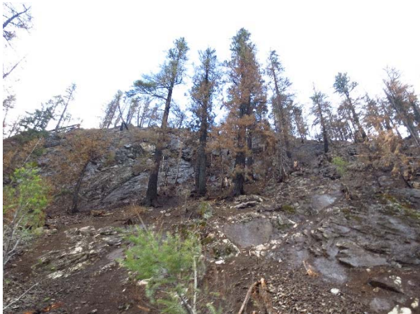
Photo 3 – Scaling and danger tree removal works at KM 41 of the Lillooet River FSR (September 3, 2015).
